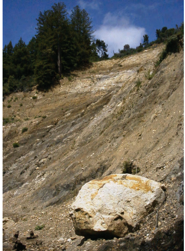
Figure 3-18. The Highland Way landslide is part of an extensive landslide complex that extends along the east side of the San Andreas Rift Valley in the upper Soquel Creek watershed. Highland Way cuts across the landslide complex and has experienced many landslide-related problems, with the latest massive landslide taking place in January, 1997 which closed the road for several years. Extensive work was conducted to remove dead trees and loose rock before the road could be repaired. This looser material is derived from Tertiary rock which consists of dark, hard, siliceous marine shale with interbedded arkosic sandstone. This sequence of marine strata forms a belt along the eastern side of the San Andreas Rift Valley for many miles extending to the south from the Highland Way landslide area.
