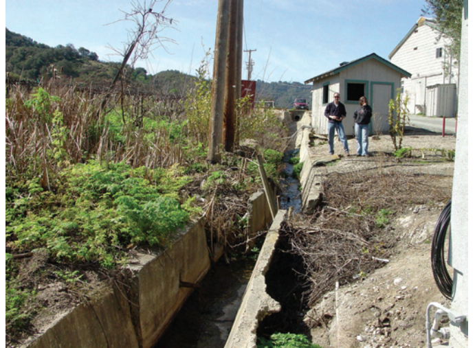
Figure 2-7. This cement-lined drainage ditch on the south side of the DeRose Vineyards shows offset from creep along the San Andreas Fault. The drain was probably constructed before the 1906 earthquake.
