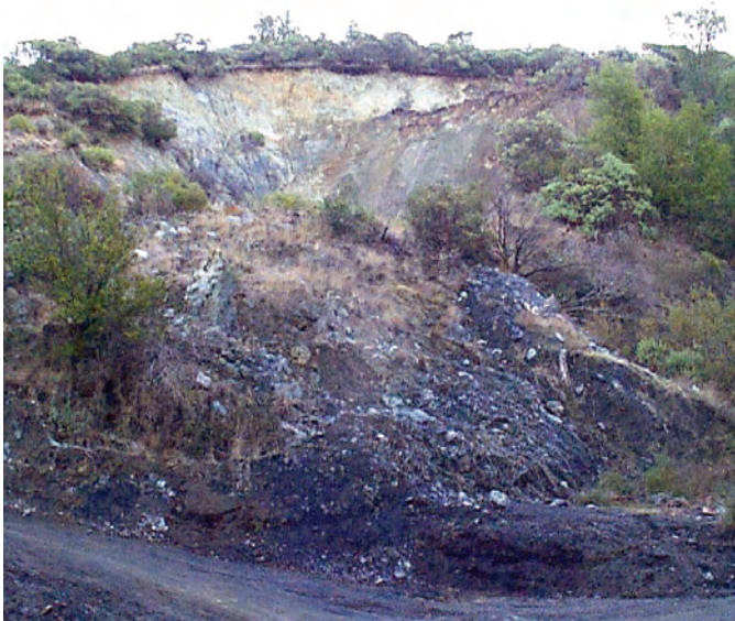
Figure 3-3. An active landslide along the Limekiln Trail causes trail closure during wet seasons. In recent winters the road has been offset by several feet. During dry months the slide area is relatively safe to examine but be aware that rocks and soil in steep slopes may be unstable from recent movement. The landslide formed in deeply weathered serpentinite, but fresh blocks of rock material have accumulated in the stream at the toe of the slump.
