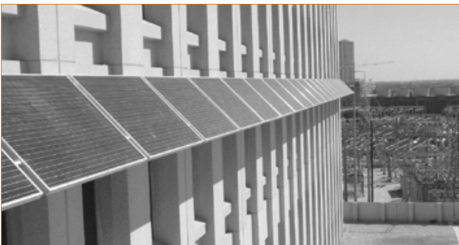
Applied Power Corporation's power modules serve as an awning for the University of Texas Houston Health Science Center. The ac modules will produce nearly 10,000 kWh of electricity each year.
