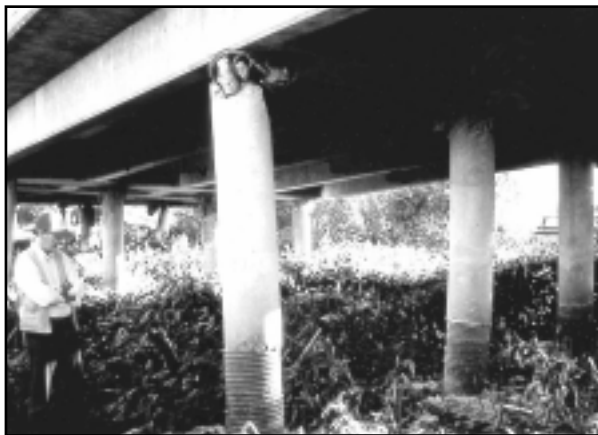
Geologist inspects settling at bridge pier due to soil compaction caused by an earthquake in California.
