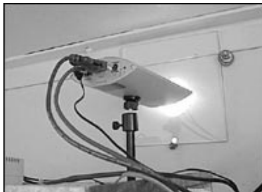
Webcam installed at streamgage shelter at Verde River near Scottsdale, Arizona.
