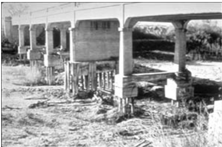
Example of bridge scour
