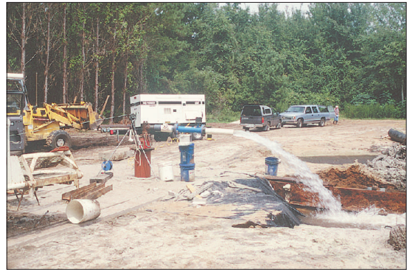
D. A public supply well in Glynn County is shown being pumped at about 1,000 gallons per minute while spinner flowmeter logs were collected to estimate percentages of water from different zones. This well is completed in the upper and lower Brunswick aquifers and the flowmeter logs help to quantify the ground-water contribution from each aquifer. Photo by Michael F. Peck, USGS.
