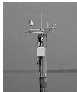
Automated real-time weather station installed over water on piling to monitor atmospheric conditions at Sneads Landing, Florida. The weather station is part of the State of Georgia's Automated Environmental Monitoring Network accessed at URL: http://www.georgiaweather.net .
