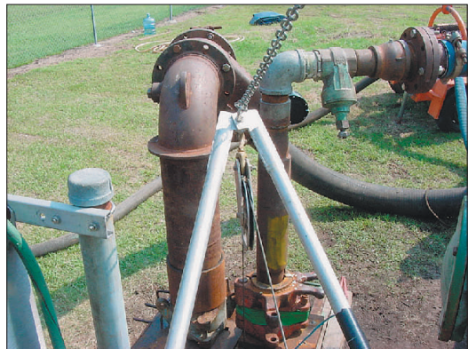
The Perry Park production well is an example of how high-chloride ground water can be withdrawn from depth with pumping. The well is located near the boundary of the saltwater plume. Here, the well is being prepared for Hydrophysical™ logging in an attempt to identify the entrance depth of the high-chloride water. Photo by Welby L. Stayton, USGS.
