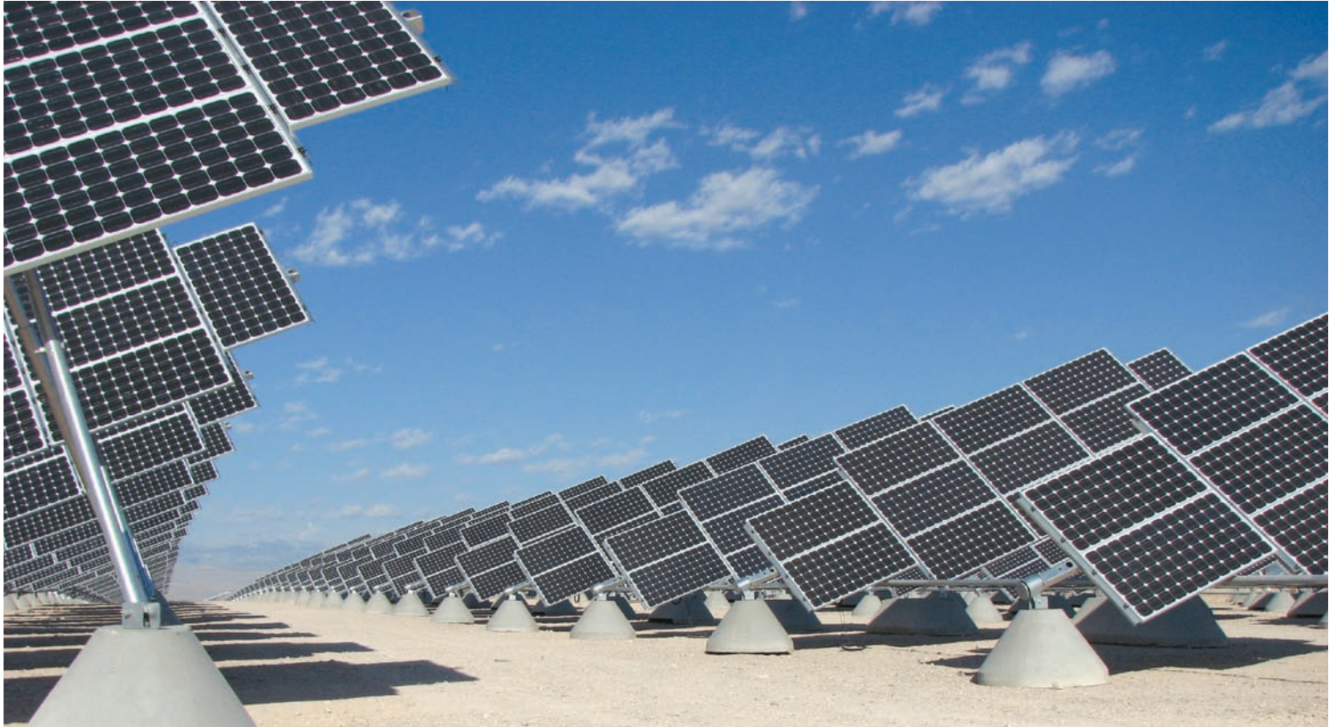
14.2-megawatt solar electric system at Nellis Air Force Base, Nevada.
