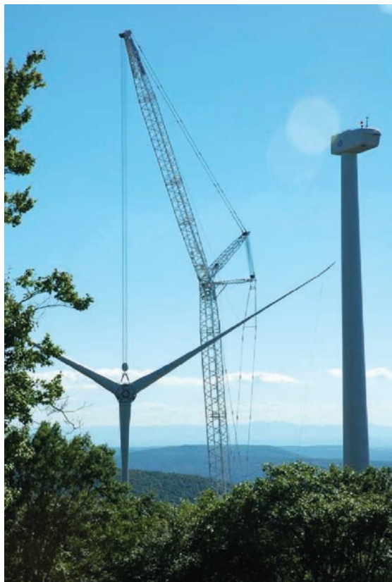
The rotor is raised on the GE 1.5sle wind turbine at Jiminy Peak Ski Area in the Berkshire Mountains of western Massachusetts. (Photo credit: Sally Wright, Renewable Energy Research Lab, UMass/PIX15160)
