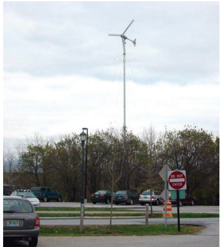
A 10-kW Bergey wind turbine installed at the University of Vermont campus in Burlington. Photo credit: Brian Killkelley
