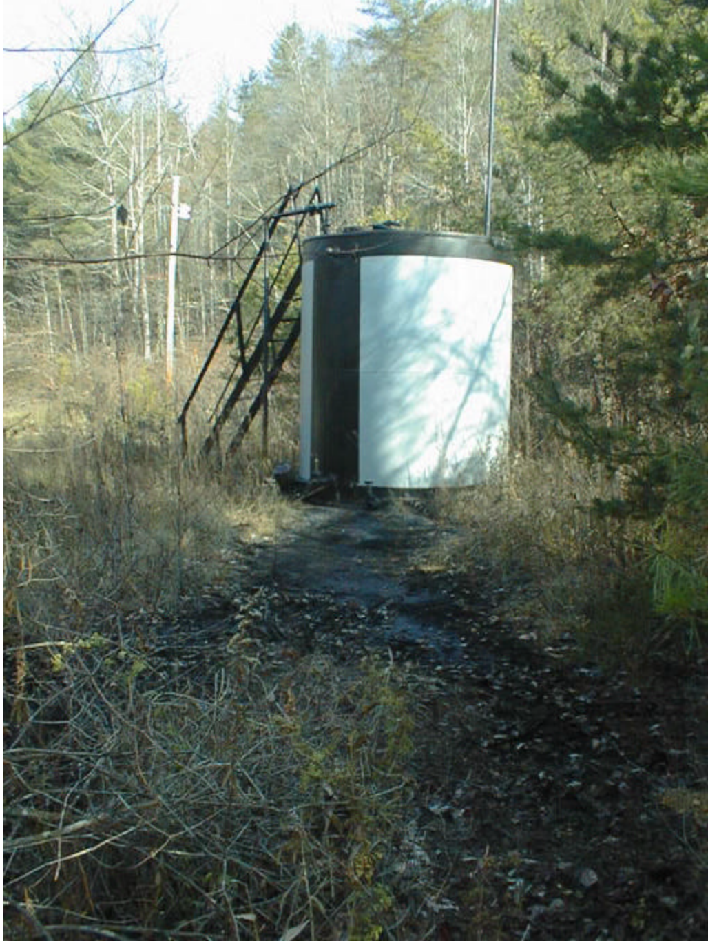
Figure 8B- View of active oil tank looking north at site BSF-1 showing spilled oil from tank on soil surface. Pit is just to the left of the view.
