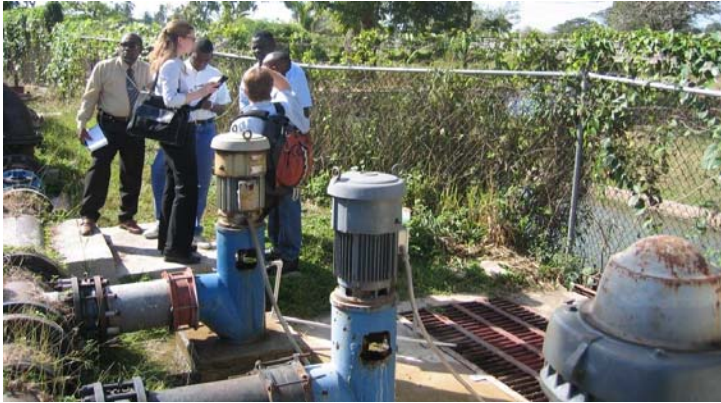
Technical site visit to water treatment facility, Spanish Town, Jamaica, 2006 for PAHO/CDC/EPA Water Safety Plan Project.
