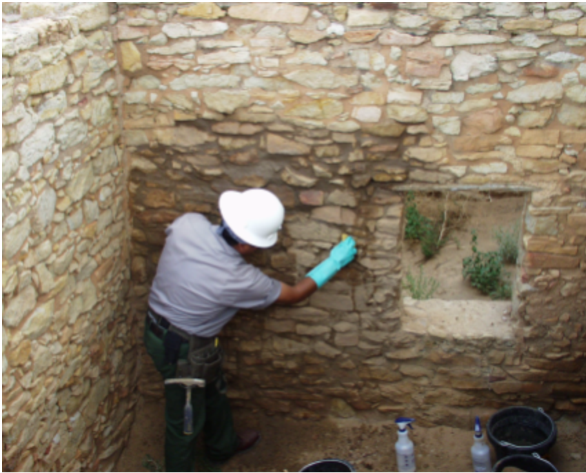
Calvin Chimoni repointing eroding masonry joints in Atsina Pueblo, El Malpais National Monument, NM.
