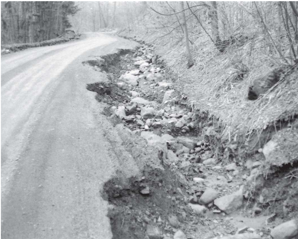
Figure 23.—Gully erosion in a road ditch. The strongly sloping and moderately steep Mardin soil is adjacent to a dirt road that has a long, steep slope.
