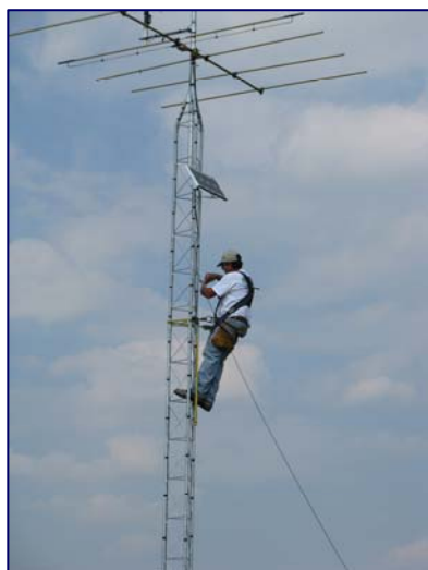
Securing tower guy wires was among the final stops in the installation of the Kansas Mesonet automated weather station at the University of Kansas’ Nelson Environmental Study Area.
