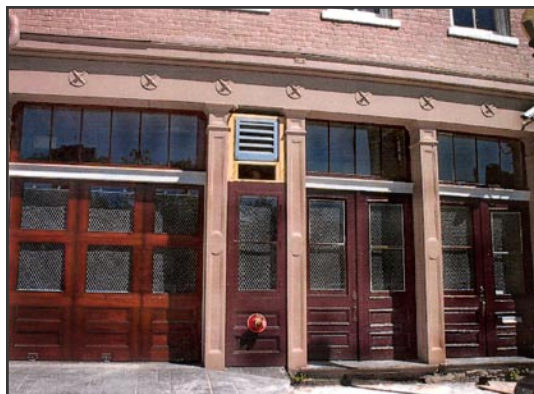
Left and Upper Right: The left bay was enlarged to create a vehicular opening which is compatible with the building's historic character.
