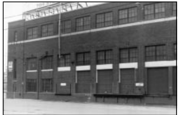
Cargo bay doors are incorporated within the fenestration rhythm. Some of the existing openings have been enlarged and later metal roll-up doors installed.
