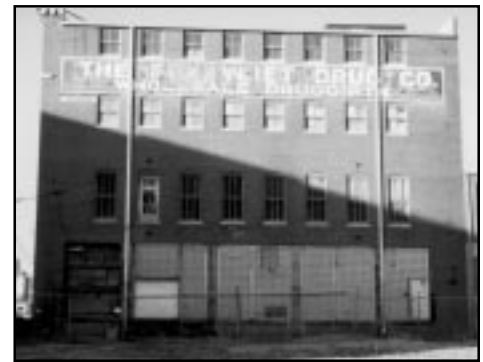
A series of cargo bay doors across the first floor is a prominent element of this facade.
