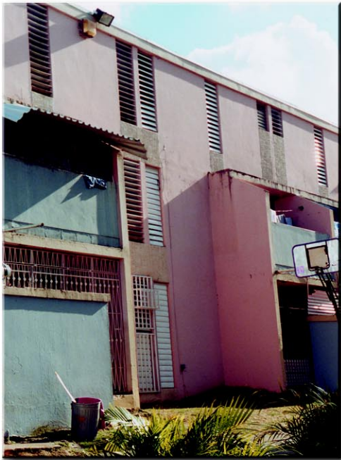
Figure 7: Examples of Health Hazards in Public Housing, Puerto Rico Public Housing Administration
