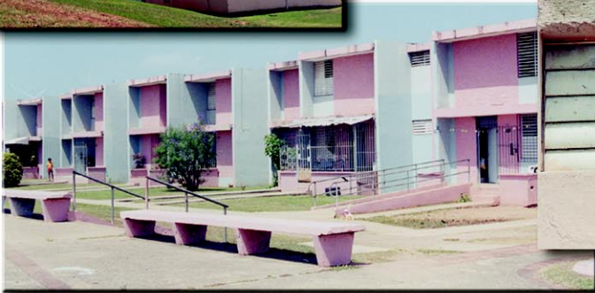
Puerto Rico Public Housing Administration, cracked walls
