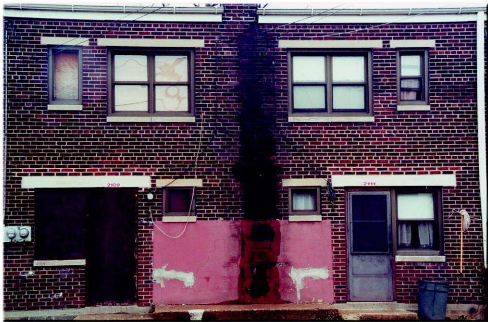
Camden Housing Authority, deteriorated structures
