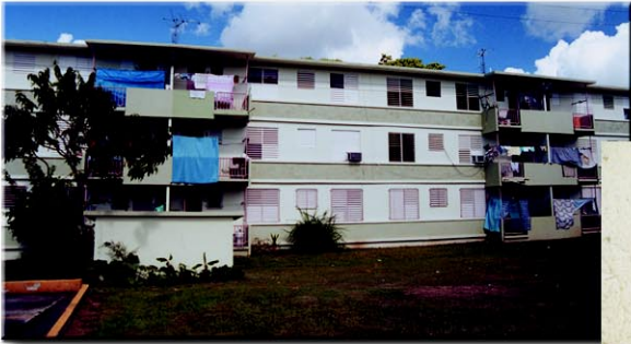
Figure 6: Examples of Deteriorated Public Housing, Puerto Rico Public Housing Administration
