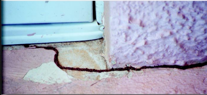
Puerto Rico Public Housing Administration, termites
