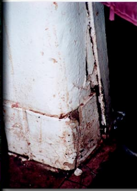
Housing Authority of New Orleans, mold and mildew
