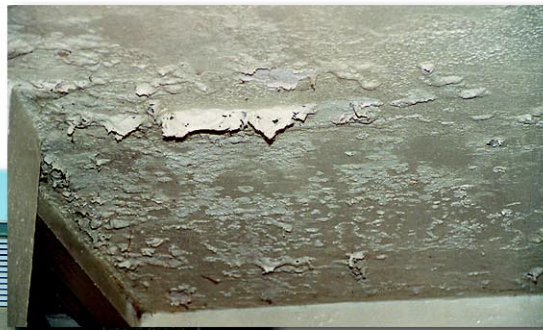
Puerto Rico Public Housing Administration, mold and mildew
