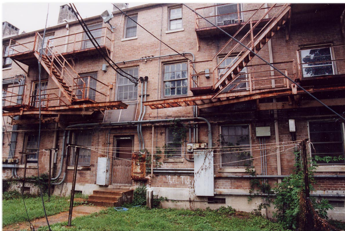
Housing Authority of New Orleans, deteriorated public housing development
