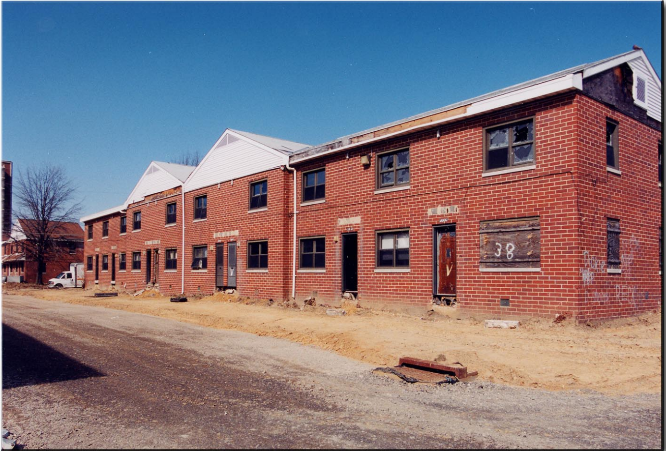
Camden Housing Authority, deteriorated public housing development
