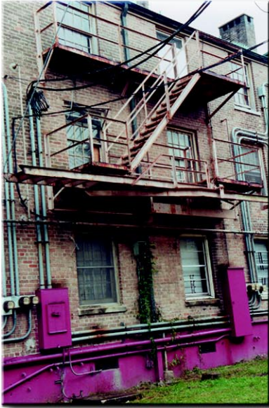
Figure 11: Examples of Public Housing Problems, Housing Authority of New Orleans
