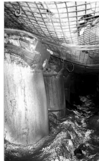
Figure 4. Standing supports, even something as strong as a Can, cannot eliminate or control floor heave
