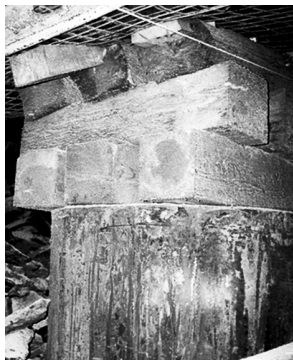
Figure 5b. If too few timbers are used, the timbers deform and control the loading of the support causing it to be less stiff than intended
