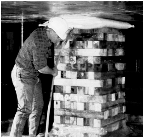
Figure 11. Prestressing of a support, such as the Hercules crib shown here, can help to offset the effects of wood shrinkage and maintain the support tight against the mine roof and floor
