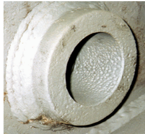
Figure 15. Corrosion of a lemniscate link bore can significantly increase the stress from link loading and increase the probability of failure
