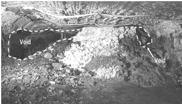
Figure 4. Cement-based remotely installed mine seal [5]. Note open void areas.
