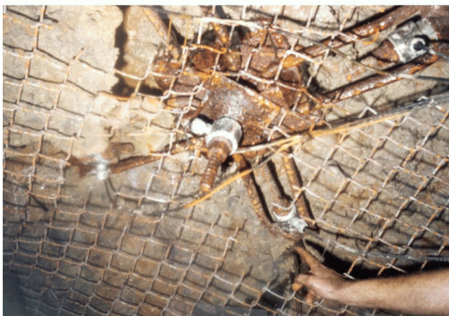
Figure 17.—Load cells at truss four-way bracket.
