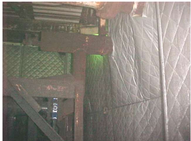
Figure 3. Barrier-absorber curtain between screen numbers 169 and 167 showing tight seal around piping.
