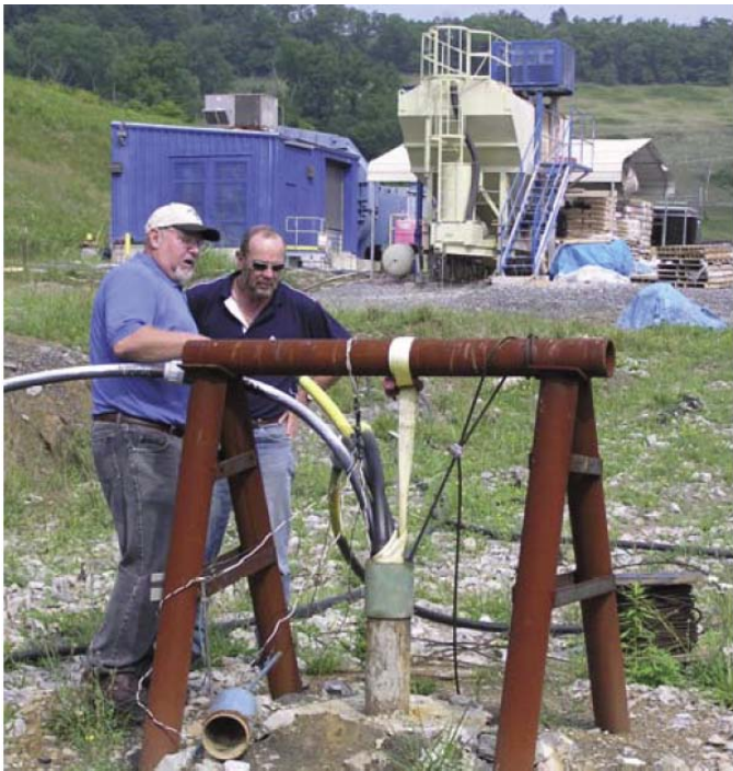
Figure 19. Cement slurries are pumped down the borehole in separate lines (pump mixing station in background).
