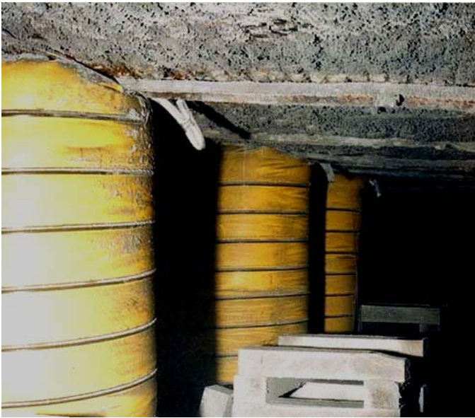
Figure 2. Pumpable roof support in longwall tailgate showing how the support can achieve full contact with mine roof.
