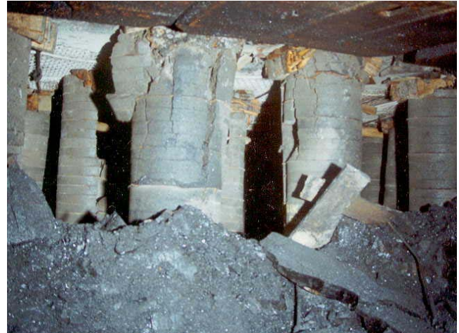
Figure 6. Failure of concrete cribbing in longwall pre-driven recovery room.
