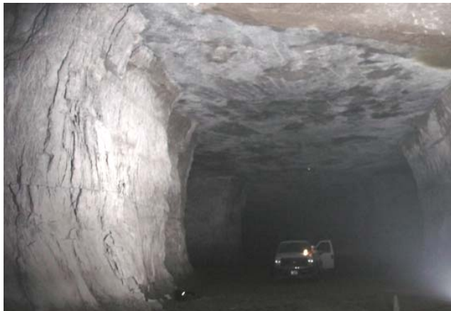
Figure 5. Example of rib slabbing and resulting concave pillar ribs that can initiate when average pillar stress exceeds about 11% of the UCS.
