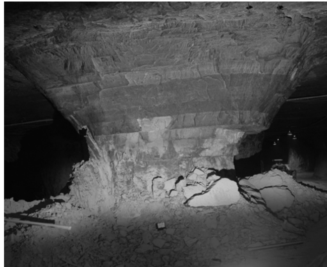
Figure 2. Pillar that has an original width-to-height ratio of 1.7 failed by progressive spalling. Thin weak beds are thought to have contributed to the failure. The average pillar stress was about 11% of the UCS prior to failure.
