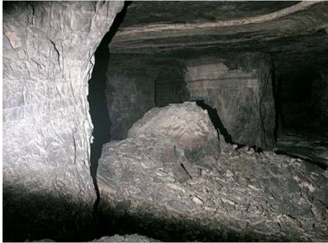
Figure 1. Remaining stump of a collapsed pillar in an abandoned area. Thin weak beds in the pillar and moist conditions are thought to have contributed to the failure. The width-to-height ratio was 0.82 and average pillar stress about 11% of the UCS.ws
