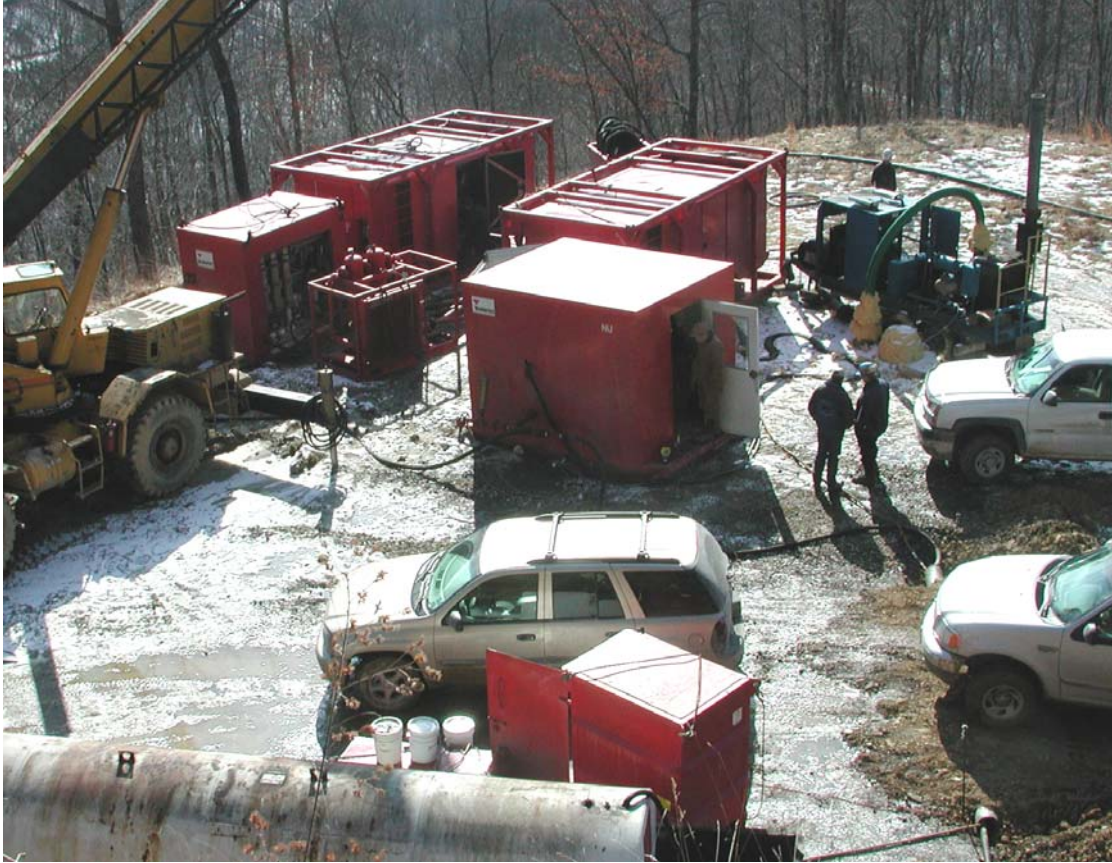
Figure 12. Nitrogen membrane separation plant.
