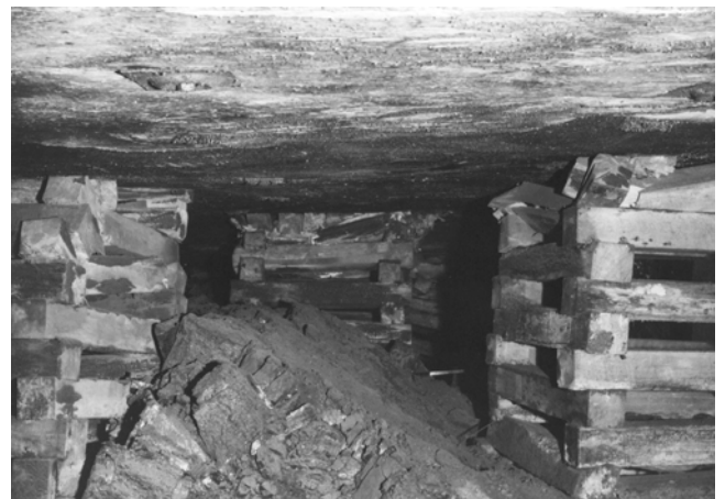
Figure 2. Excessive pillar line floor heave.
