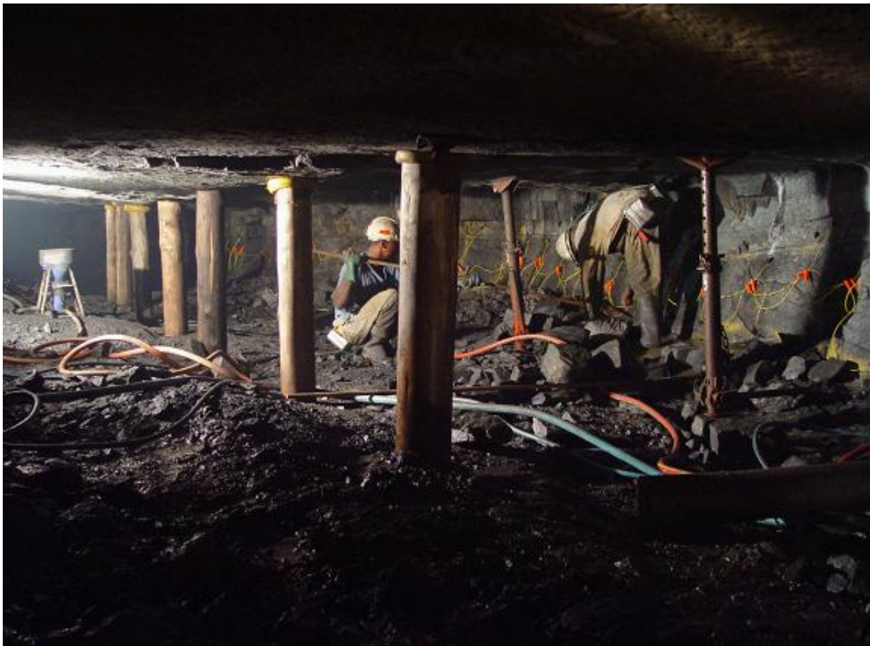
Figure 7: Prestressed props can be employed along face line as they can withstand the ground reaction and force from the blasting at the face.
