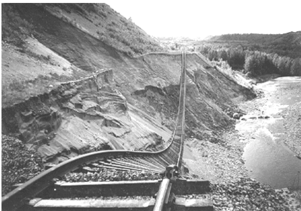
Figure 6. Rail track demolished by a slope failure.
