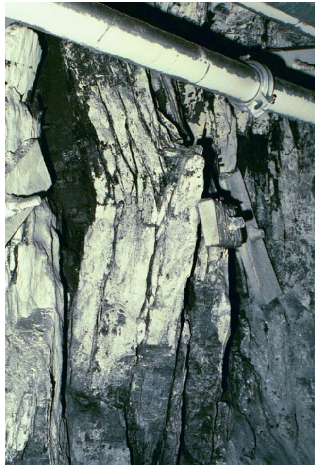
Figure 2. Photograph illustrating rib failure by buckling.
