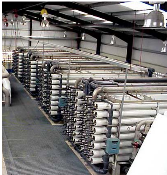
Figure 3-16. Banks of RO vessels in a seawater desalination plant
