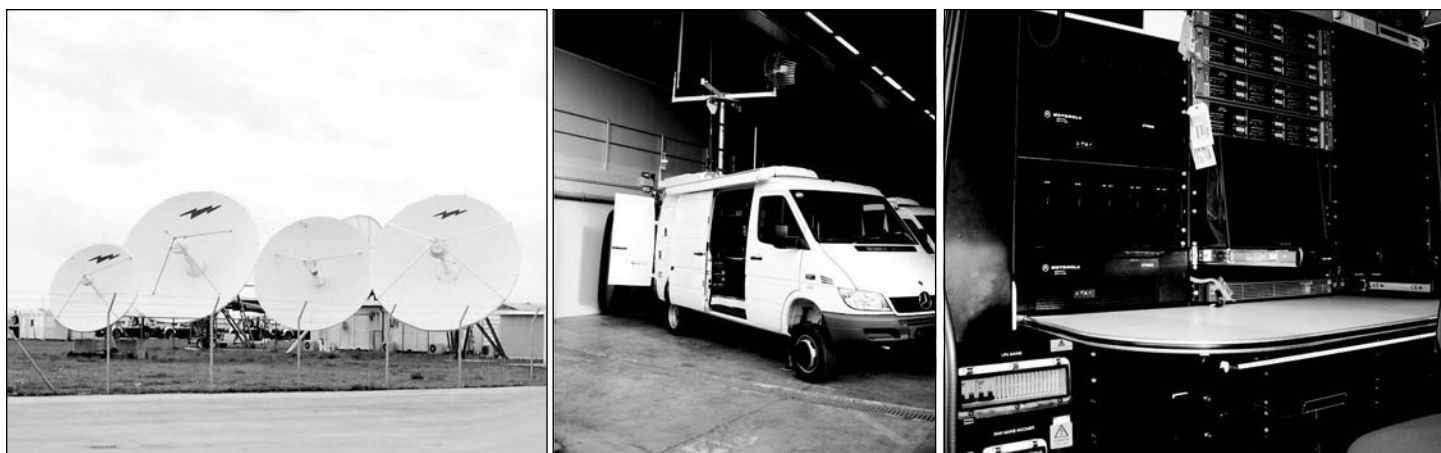
Figure 4: UNLB's Communications and Data Facilities
