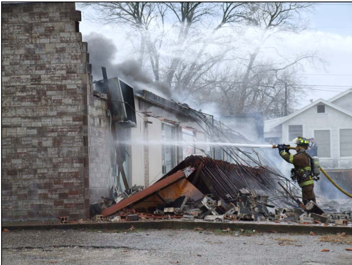
Photo 2. View from North end of building – post collapse. Photo courtesy of fire department.
