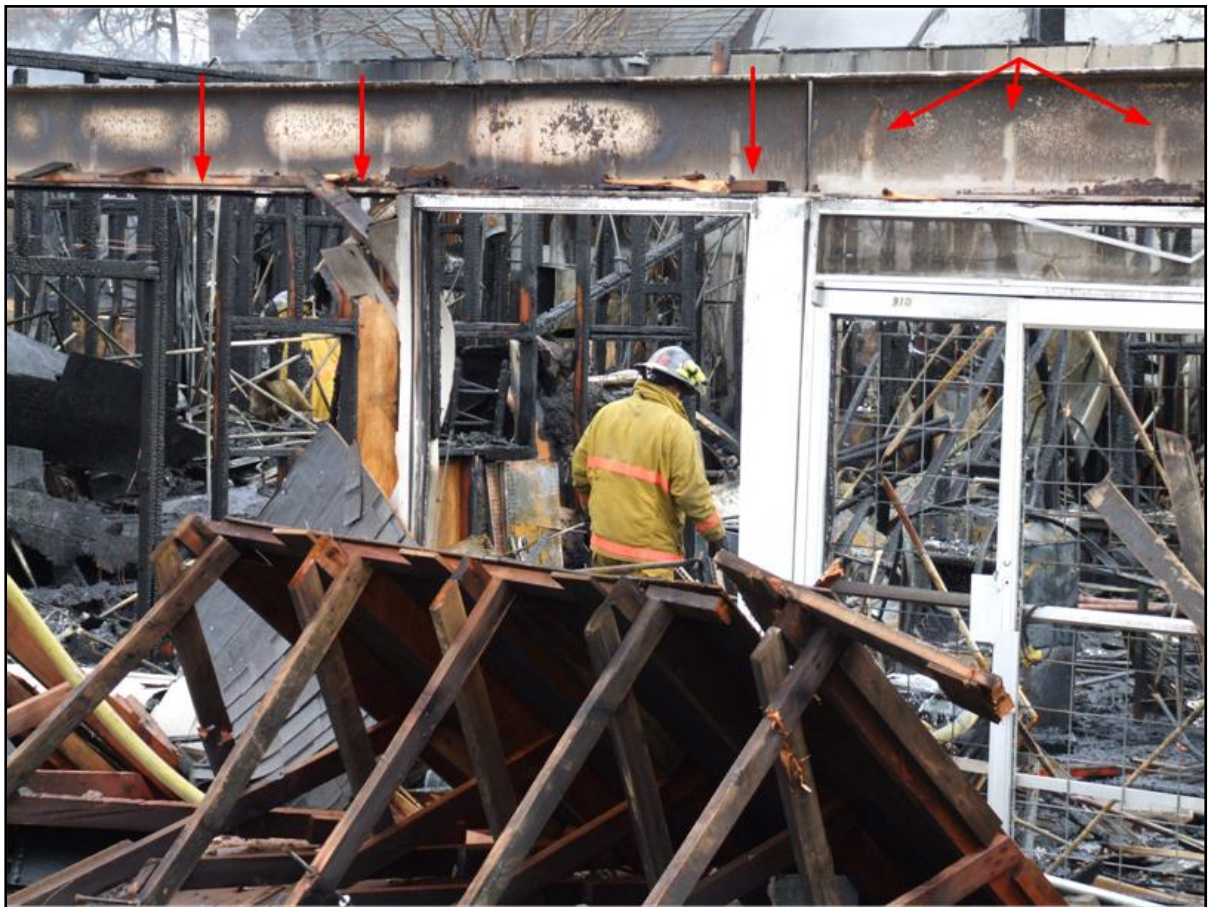
Photo 3. Note steel I-beams running across front wall above windows and doors. Note wood fragments where awning frame was connected to the I-beam. Burn patterns also indicate location of awning frame. Photo courtesy of fire department.
