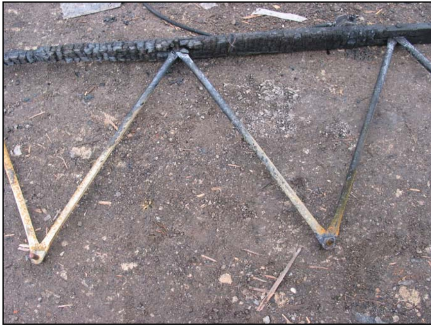
Photo 5. Open-web pin-connected trusses after fire. Photo courtesy of fire department.
