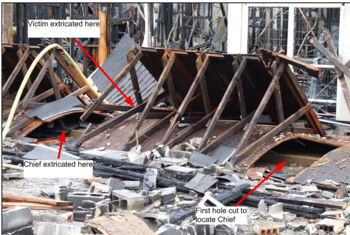
Photo 7. Awning after collapse. Note holes cut through awning during extrication to free the trapped fire fighters. Also note how curvature of awning creates a void underneath Photo courtesy of fire department.
