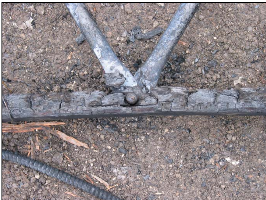
Photo 6. Close-up of pin connection in open-web pin-connected trusses Photo courtesy of fire department.
