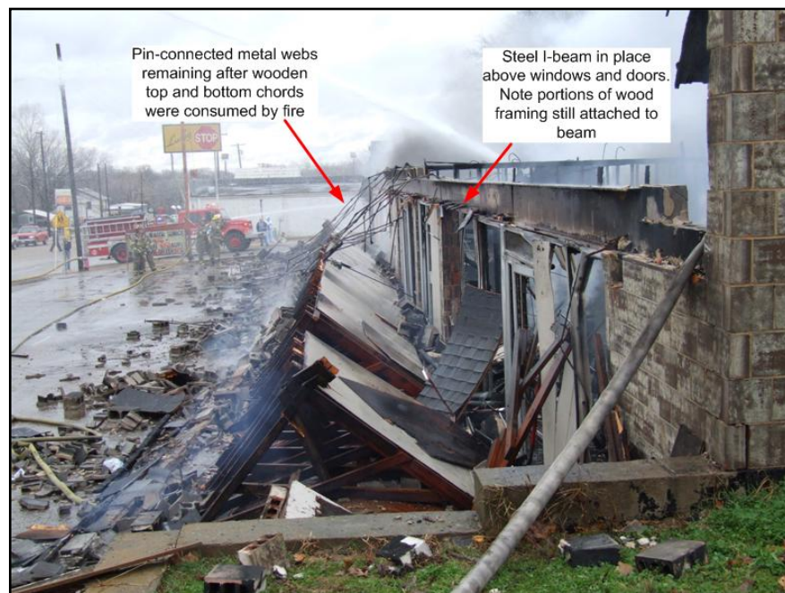
Photo 4. View from south-end of structure after awning collapse. Note the pin-connected metal webs still connected to the awning. The top and bottom chords of the trusses have been consumed by the fire. Also note the steel I-beam in place above the windows and doors. Refer to Figure 3 and Photos 5 and 6 for more details of the truss construction. Photo courtesy of fire department.
