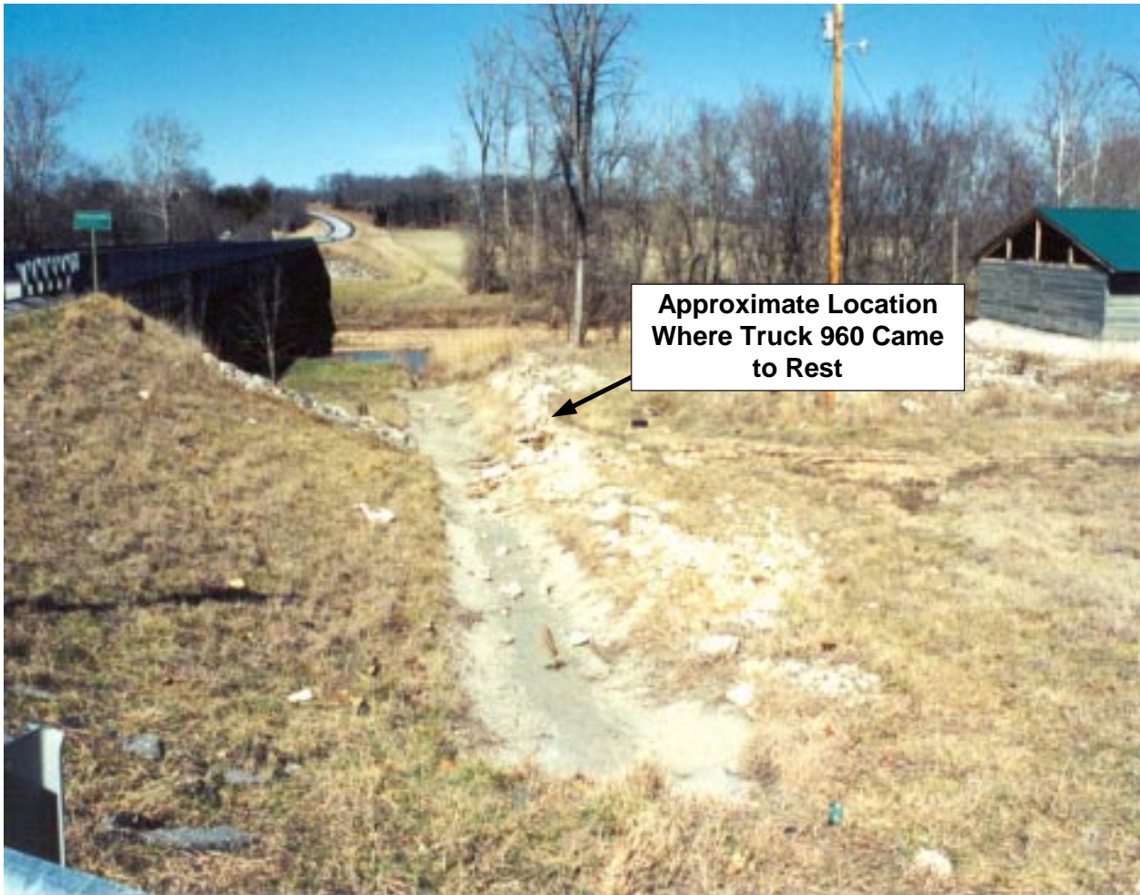
Photo 3. Concrete Culvert Where Truck 960 Came to Rest
