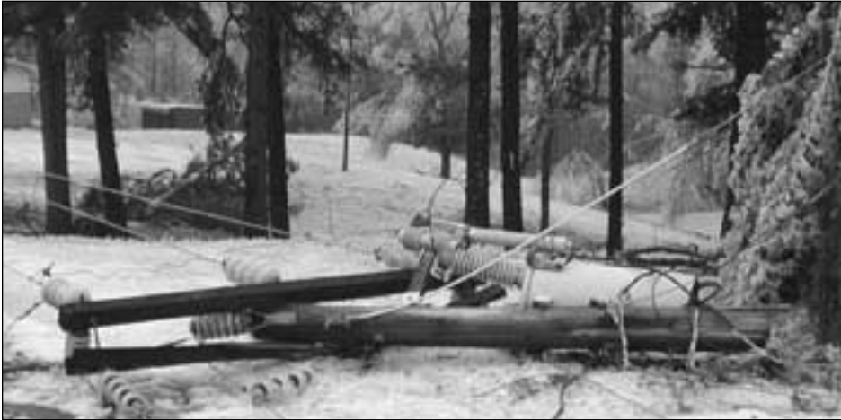
Downed lines and electrical poles blocked icy roads and caused massive power outages throughout the state during the recent Arkansas ice storm.
