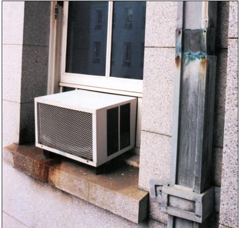
Figure 3: One Of About 250 Inefficient Window Air Conditioning Units in the Dwight Eisenhower Building in Washington, D.C.
