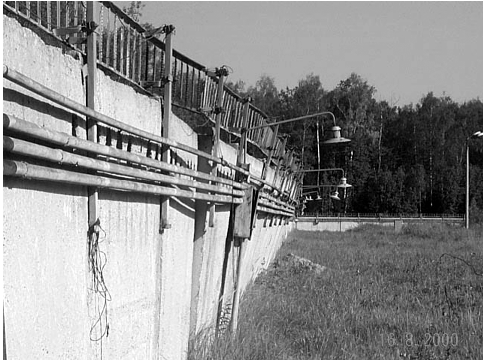
Figure 5: Unstable Perimeter Fence at a Biological Site in Russia, before Security Upgrades
