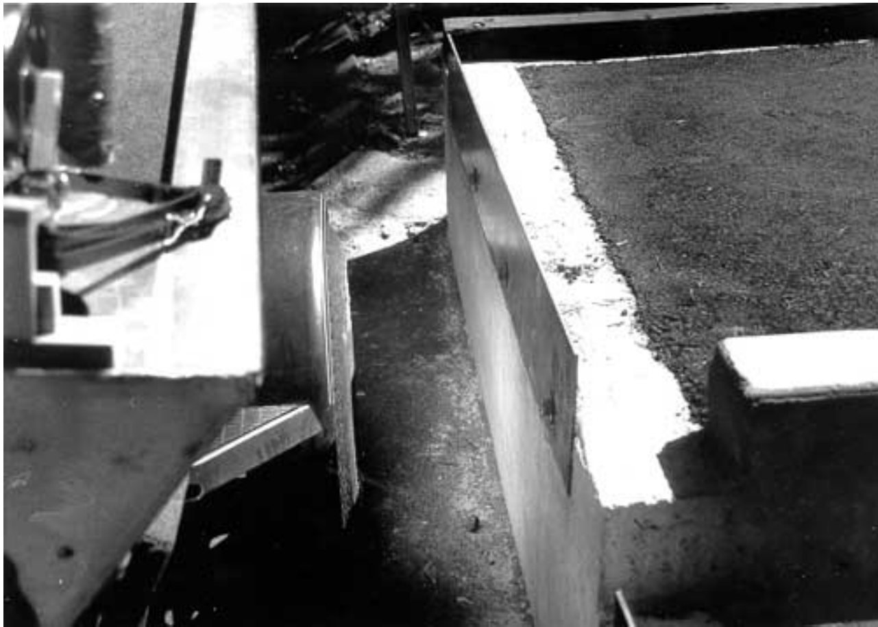
Figure 6 - The 1/4 inch steel plate on the end of the platform allows boat trailers to get close to the platform while preventing wheelchairs from rolling off.
