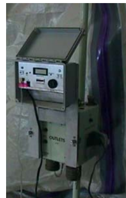
Pressure gauge with differential pressure alarms
