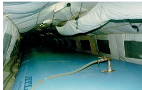
CB hardened water distribution system
