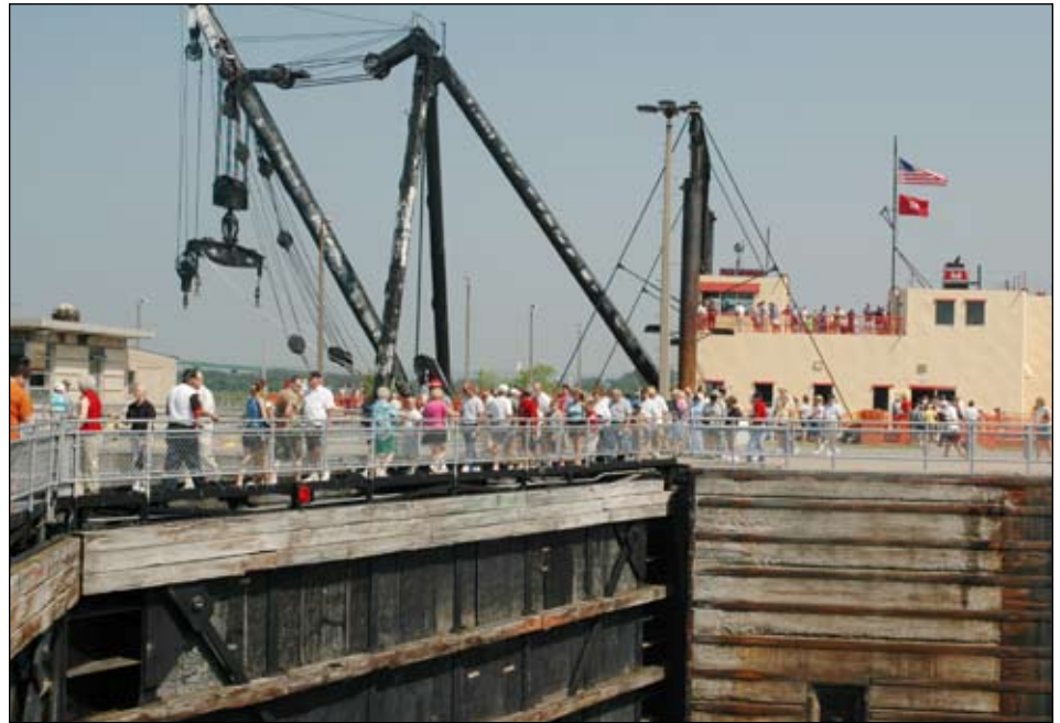
Gates, like the ones pictured above, wouldn't proper miter closing, the Poe Lock for two hours Sept. 24. But Soo Area employees troubleshot the problem and got the lock working properly.
