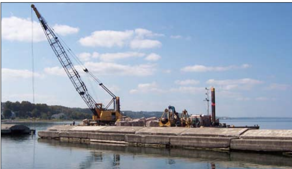
Detroit District employees made a commitment that awarding all its contracts – like the one to repair the Petosky breakwater pictured above – would be a priority in order to make the fiscal year deadline on Sept. 30.
