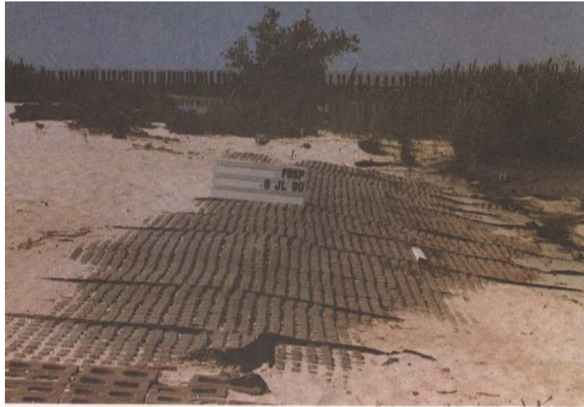
Figure B-6 Ercomat Revetment
