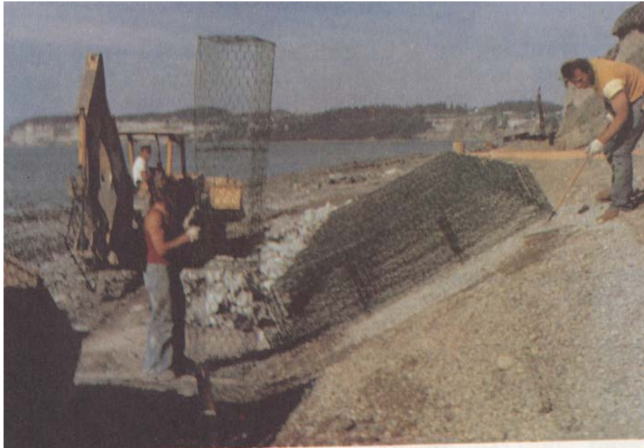
Figure B-14 Unfilled Gabions
