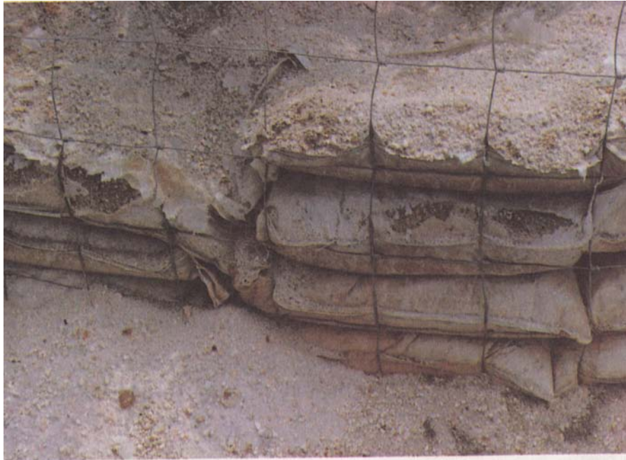
Figure 37 Deteriorated Sand Bag (June 1979)
