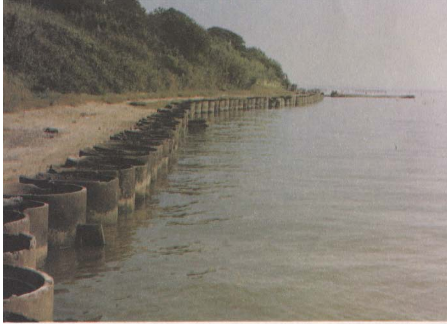
Figure A-12 Used Concrete Pipe Bulkhead
