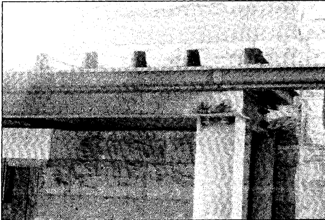
Figure 5.8: Detail of steel structure at northwest areaway roof with failing paint and rust bloom. The K-type hanging gutter and downspout are also experiencing paint failure.
