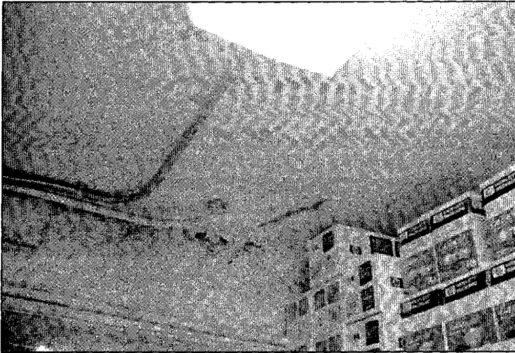
Figure 5.19: Detail of paint failure and water infiltration at concrete ceiling of north storage room. The painted concrete and brick wall at this location has also eroded and is showing signs of rust bloom from embedded ferrous elements.
