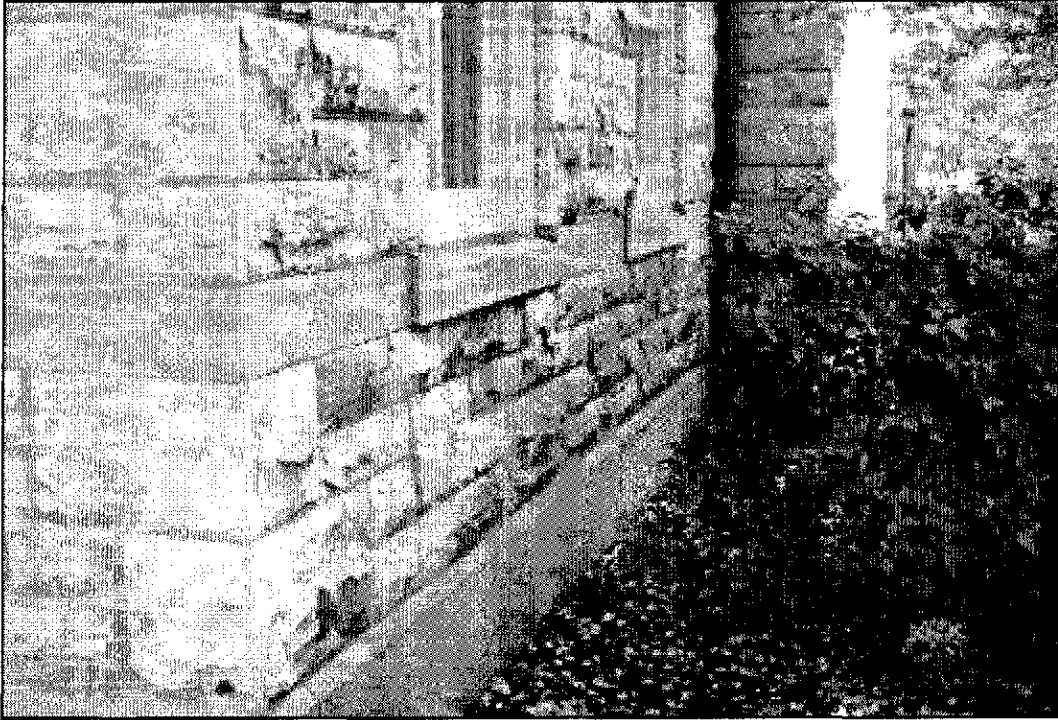
Figure 5.12: Northeast elevation with significant biological growth on underside of rock-faced finish marble and granite water table.
