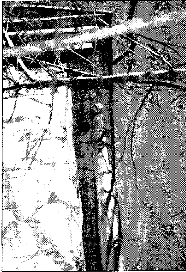
Figure 5.14: Detail of through-cornice downspout disconnected from rain leader at south end of southeast elevation. The downspout is clogged with branches and foliage.
