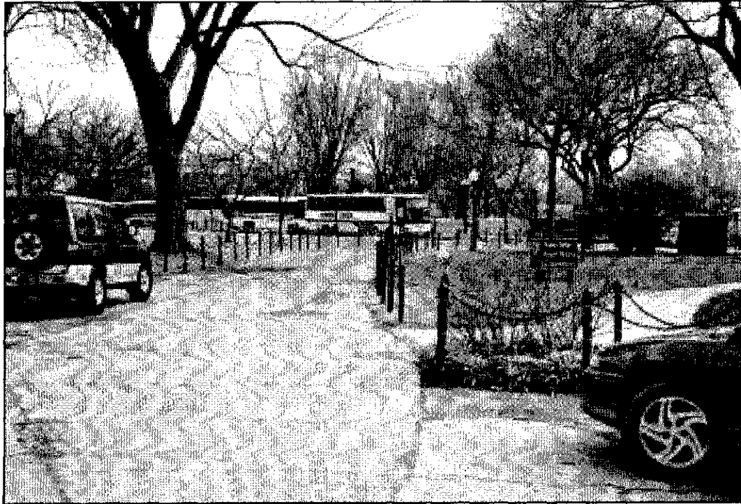
Figure 5.1: Asphalt service drive north of lodge, view to the southeast with serious cracking and previous patches evident.
