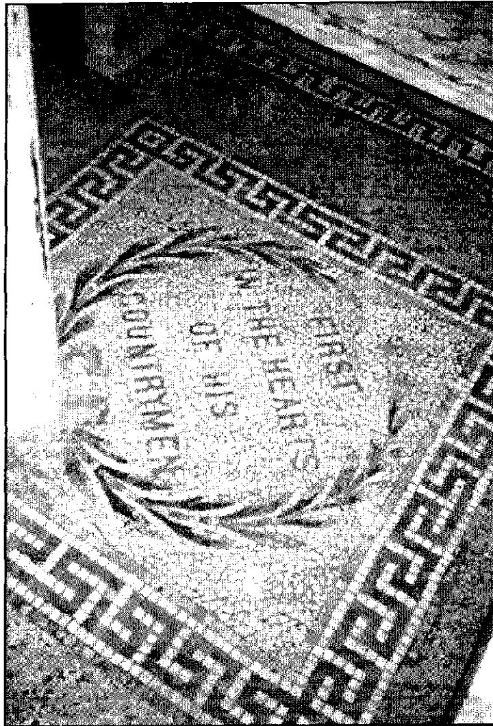
Figure 5.20: Washington Monument, south corridor, west terrazzo panel.
