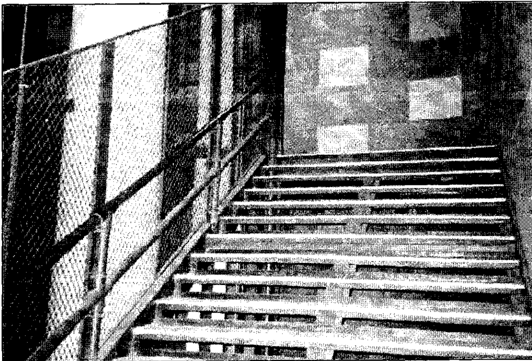
Figure 4.36: Stair to 260-foot level, with marble headers and granite stretchers in background.
