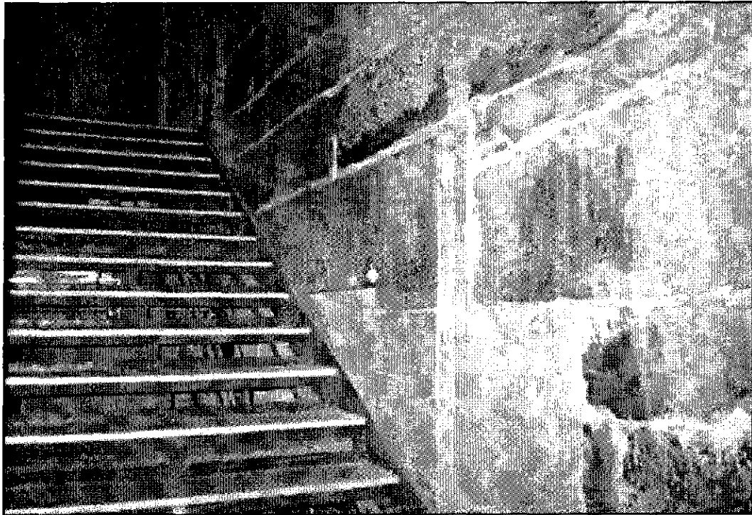
Figure 5.17: Washington Monument, interior, central shaft, discoloration of gneiss at 15-foot level.
