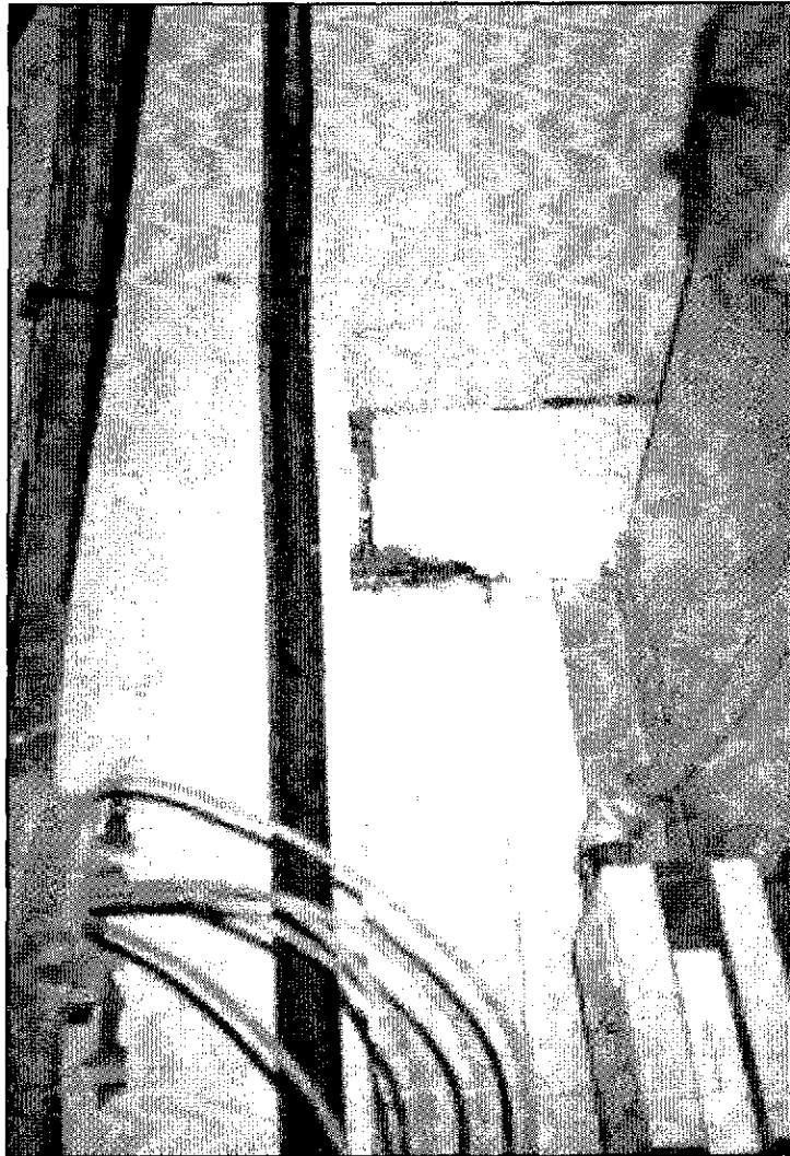
Figure 5.23: Washington Monument, Bunker 1, interior, mechanical room, north wall, rusting louver.
