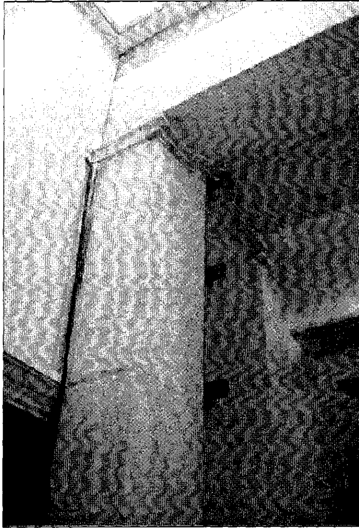
Figure4.28: East elevator lobby, view to the east, showing the glass transom to the east portal and the surface-mounted conduit penetration. Also note the rough-finished stone courses above the door surround.
