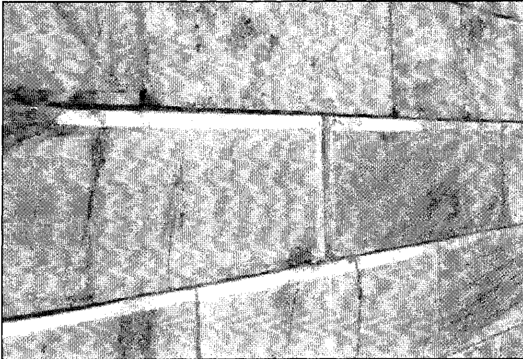
Figure 5.8: West elevation with original tool marks evident around perimeter of stones. There are also areas of red or pink staining indicating locations of inclusions in the marble.
