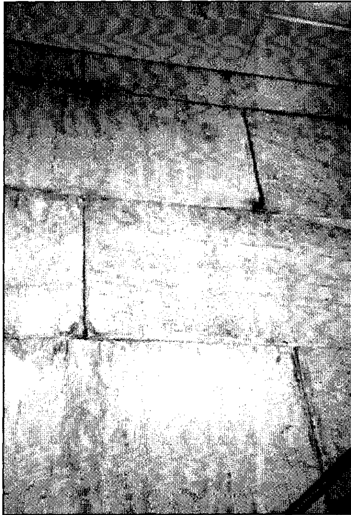
Figure 5.13: Washington Monument, interior, central shaft, open joints at 490-foot level stairs.
