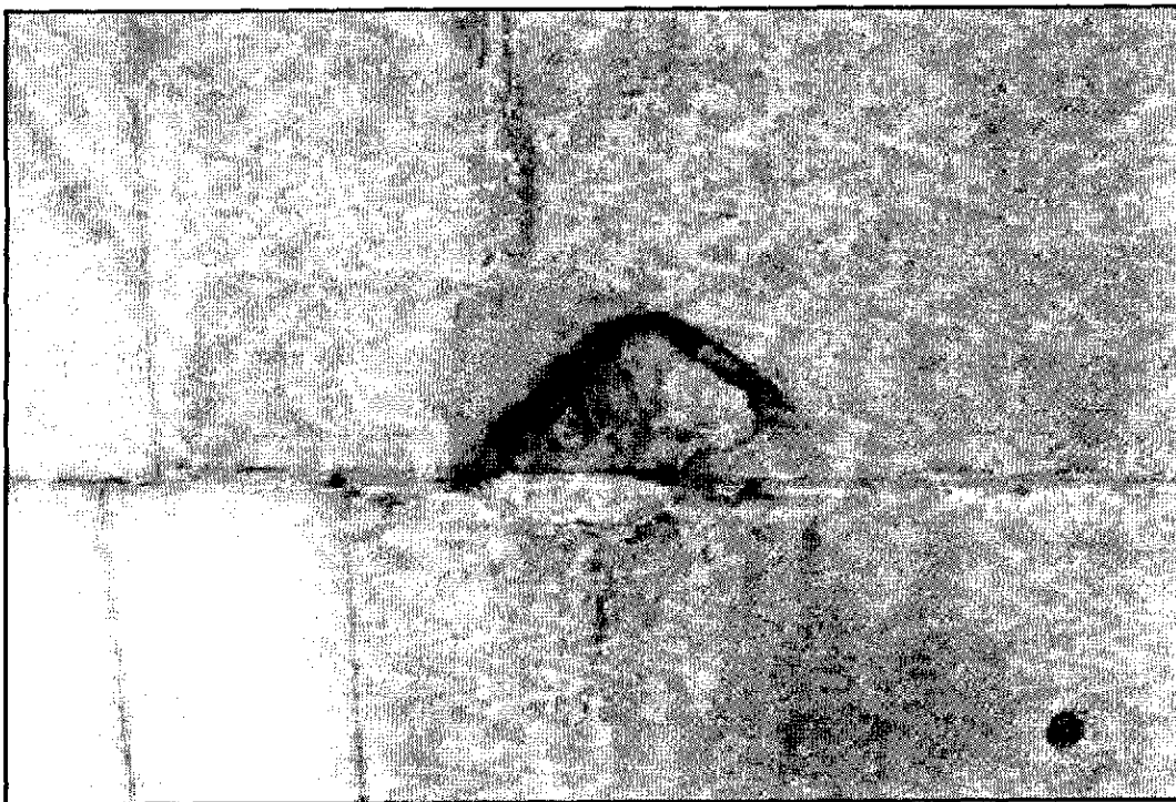
Figure 5.7: North elevation near ground level with failed patch. It appears that moisture behind the patch was supporting biological growth before the patch completely failed.
