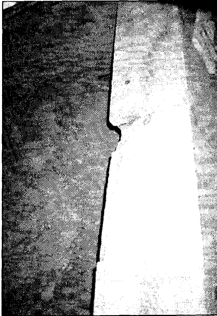
Figure 5.12: Washington Monument, interior, central shaft, spall on pier at 480-foot level.
