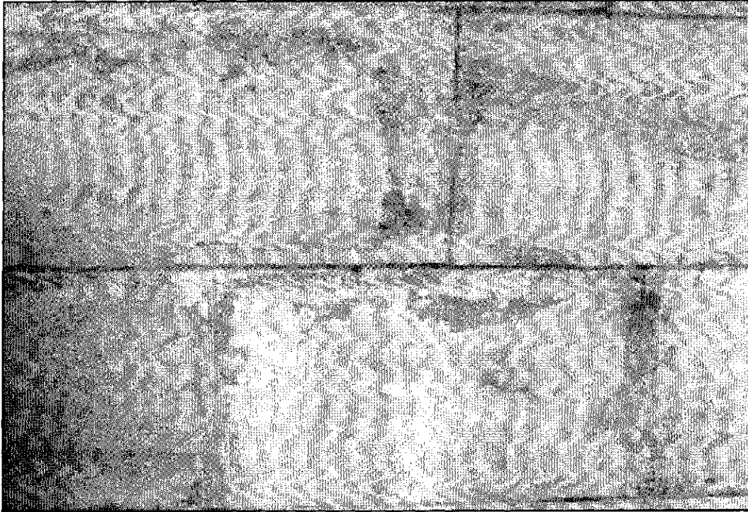
Figure 5.5: West elevation patches near ground level. The patch material absorbs and evaporates water at a rate that is very inconsistent. Dark areas of the patch are still damp hours after the last rainfall, which gives the patch a mottled appearance.
