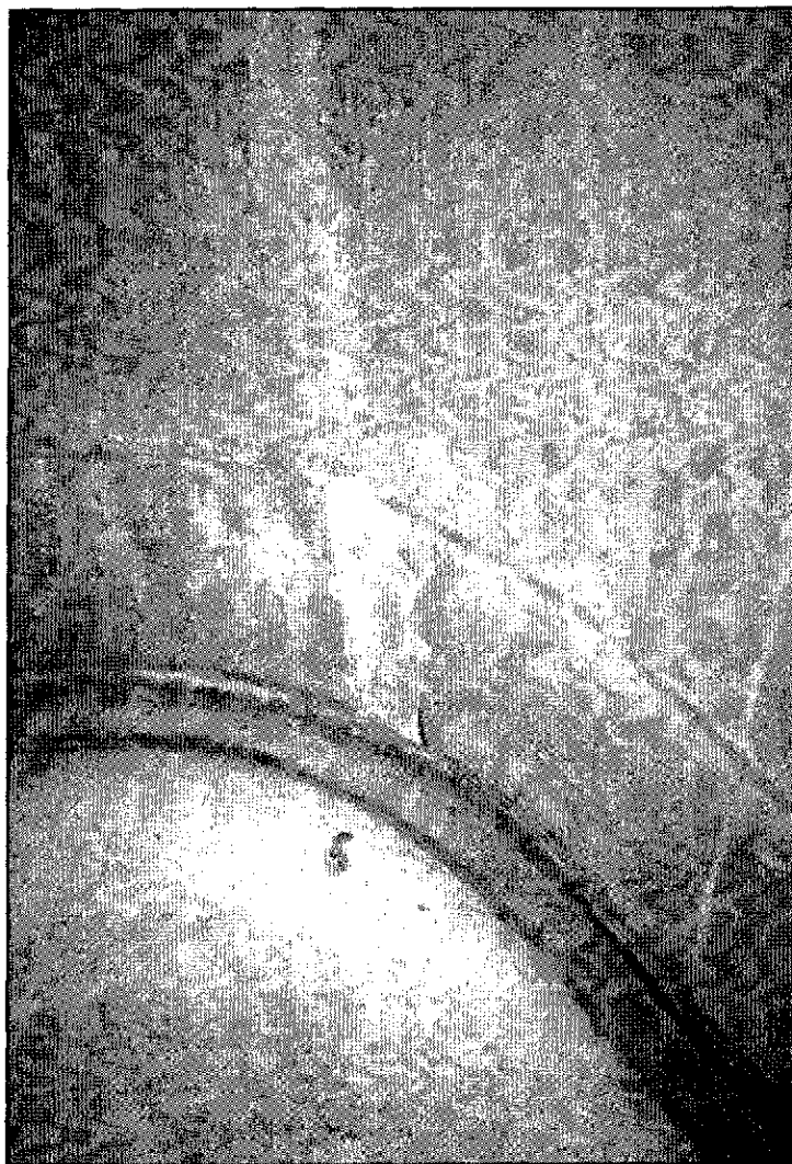
Figure 5.11: Washington Monument, interior, central shaft, delamination at corner stones.
