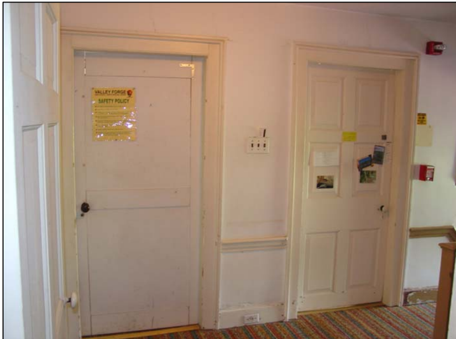
Figure 60. Room 201 (second- story stair hall), west wall, showing the original six- panel door to Room 202 (right) and the plywood replacement door to Room 203 (left). Note the doorway trim and the original chair rail.
