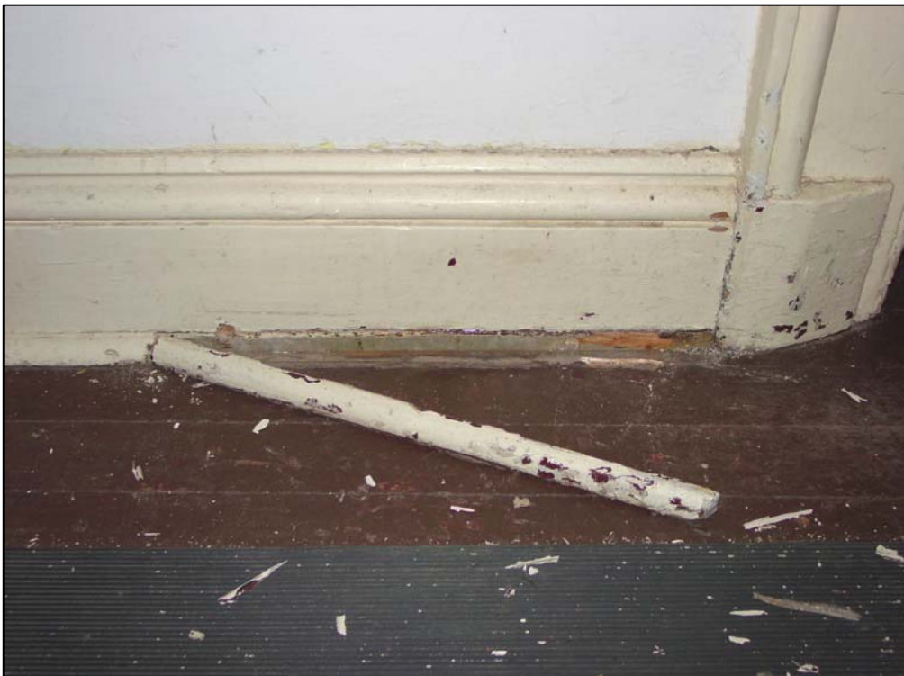
Figure 53. Room 103 (original kitchen), typical baseboard used in the house, with toe molding added when the current floor was installed.
