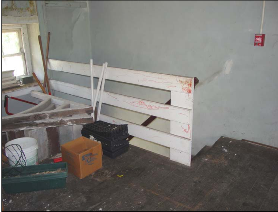
Figure 84. Room 207 (second story of the ell), northeast corner, railing along the stairwell of the stairway down to Room 104 (first story of the ell).
