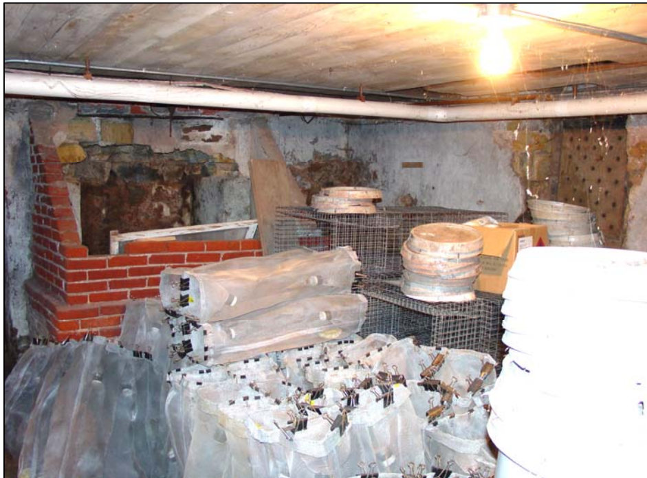
Figure 33. Room 001 (north basement), showing added ash box at the west wall and an original window at the north wall. Note also the board ceiling.
