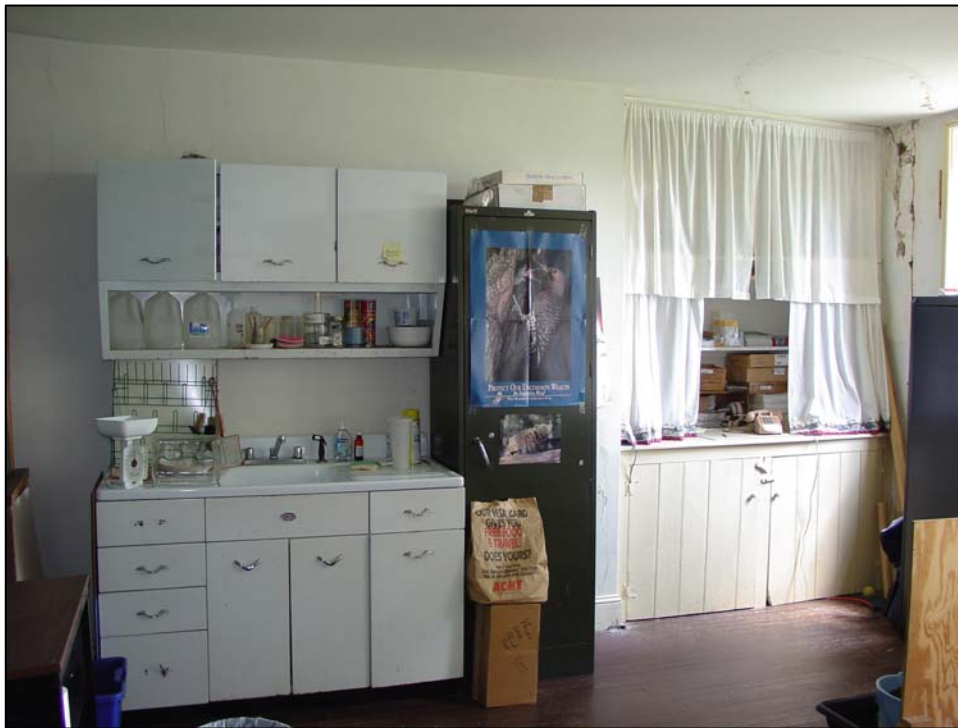
Figure 49. Room 103 (original kitchen), east wall, showing the cabinetry at the south end of the wall.
