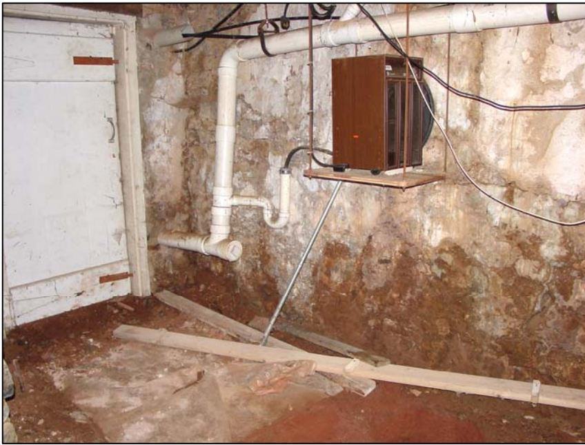
Figure 35. Room 002 (south basement), southeast corner, showing the narrowed bulkhead doorway, along with a later dehumidifier and drain pipe.
