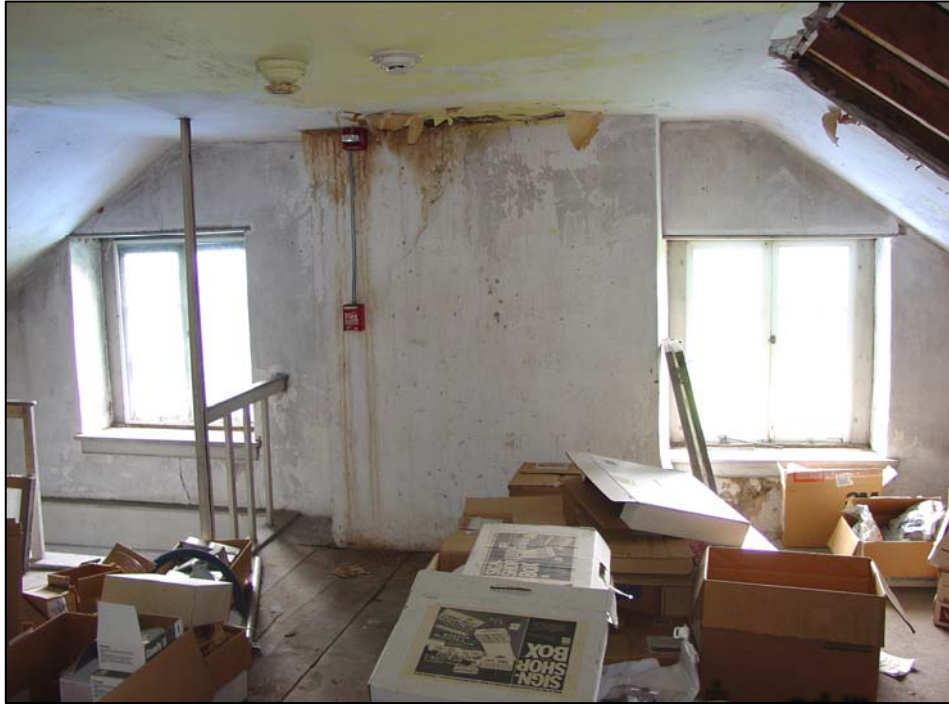
Figure 85. Room 301 (east attic room), east wall, showing windows flanking chimney, and stairway to Room 205 (southeast bedroom).
