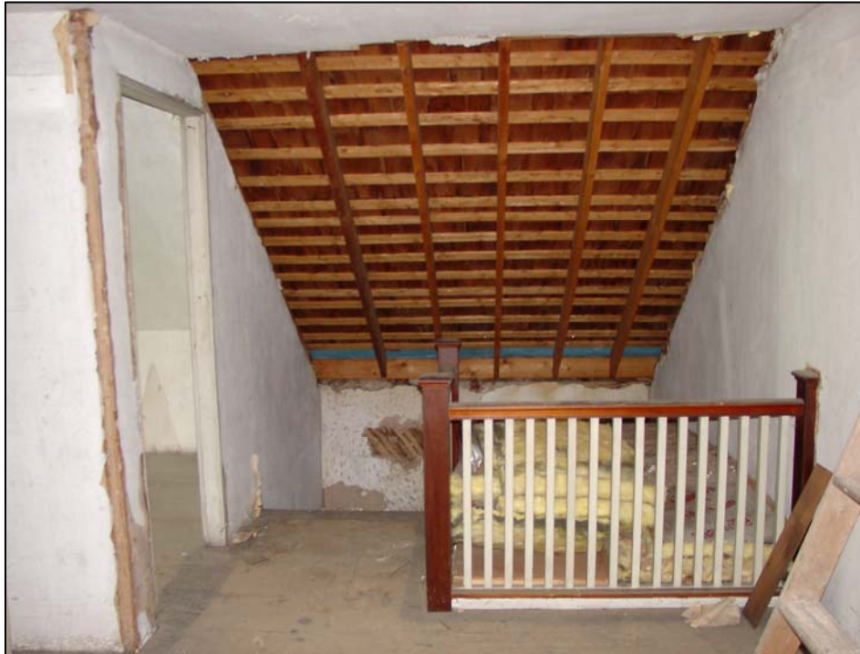
Figure 88. Room 302 (center attic room), looking north at the center stairway and the replacement balustrade. Also shown are the doorway to Room 303 (northwest attic room) at left, and an area of ceiling disturbed by the addition of an early 20 th - century dormer (removed in 1978).
