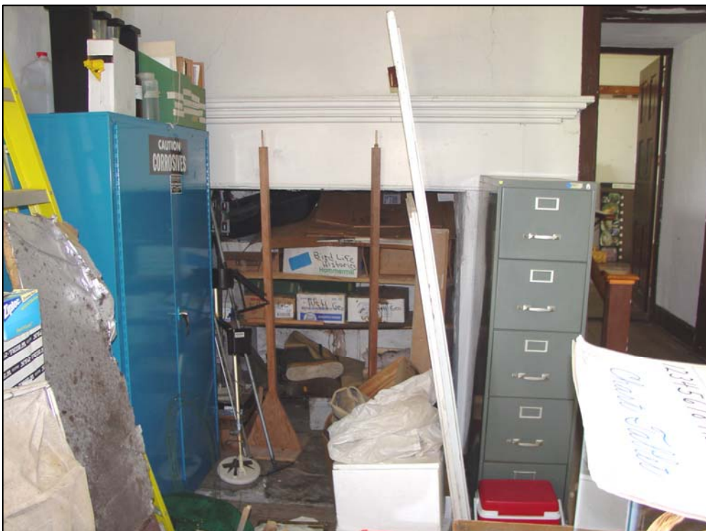
Figure 59. Room 104 (first story of the ell), west wall, showing the fireplace fitted with shelves for storage.
