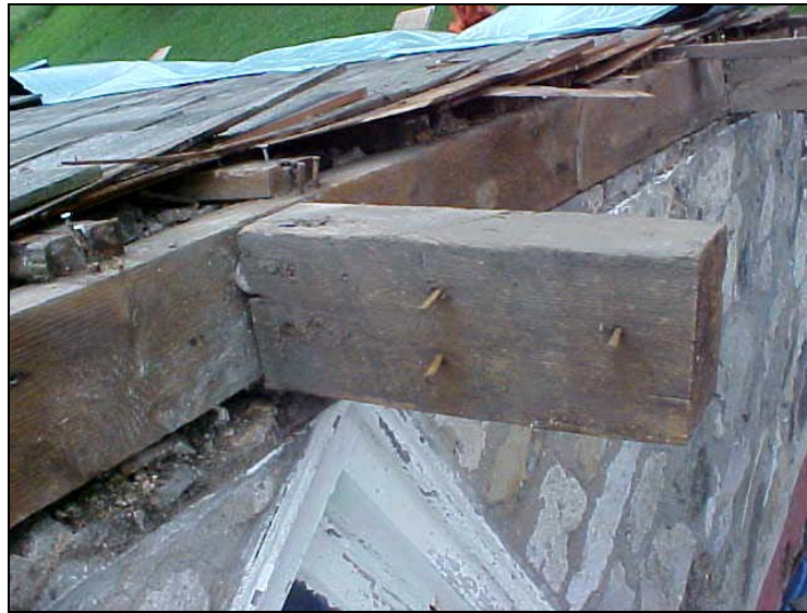
Figure 11. Nonoriginal eave extension, or "outlooker," mortised into original gable end rafter (2004 photograph).
