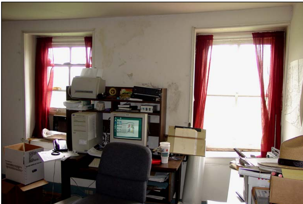
Figure 80. Room 206 (southeast bedroom), south wall, showing some deflection due to the insertion and later removal of the bay window in the first story of the house.
