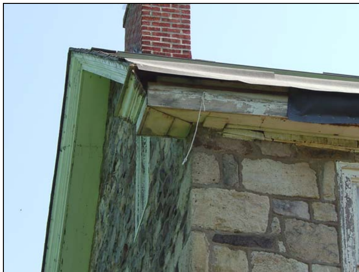
Figure 12. Detail of cornice and eave configuration, which likely dates from ca. 1840- 1860 (2004 photograph).
