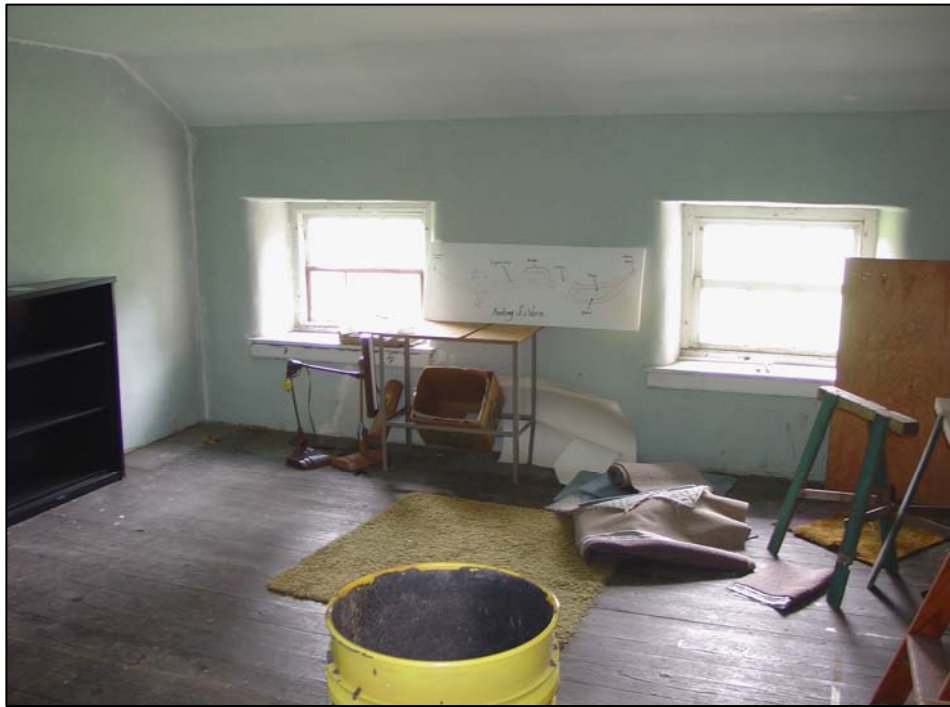
Figure 82. Room 207 (second story of the ell), south wall, showing windows with three- over- three, double- hung sashes and curved window reveals typical of ca.- 1840s construction in the area.
