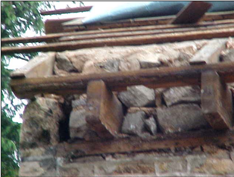
Figure10. Roof framing details, direct view: rafter ends sit on a plate, which is carried by the attic floor joists, which sit on a second plate (2004 photograph).
