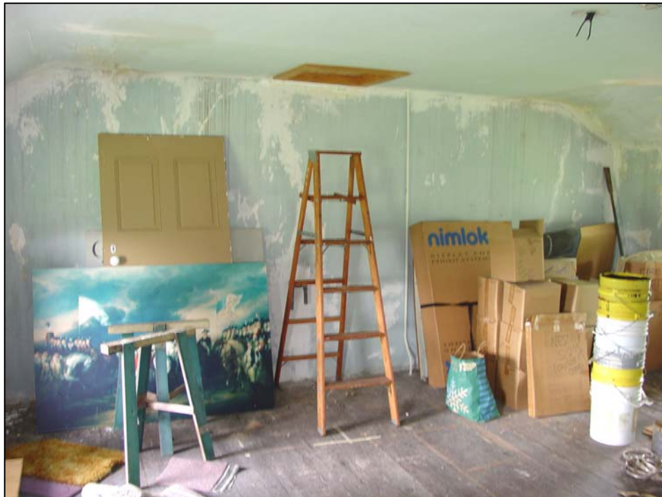
Figure 83. Room 207 (second story of the ell), looking west and showing the ell's attic scuttle.
