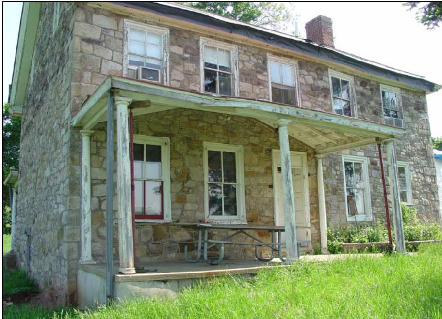
Figure 20. Front porch of house, added ca.1860- 1880, and modified with Tuscan- order columns ca. 1902- 1919.
