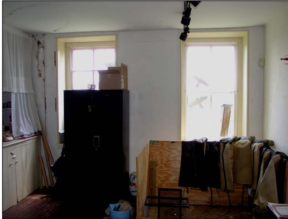
Figure 50. Room 103 (original kitchen), south wall (largely reconstructed after the removal of the bay window).
