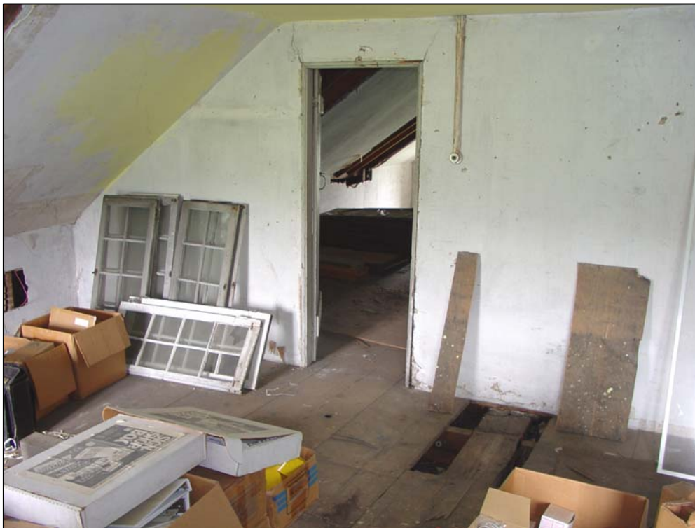
Figure 87. Room 301 (east attic room), west wall, showing the doorway to Room 302 (center attic room).
