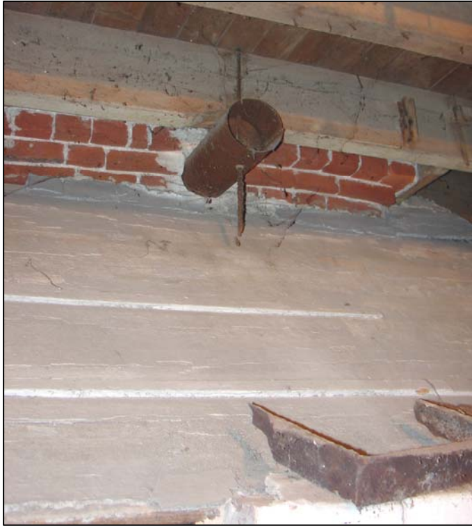
Figure 17. Duct with damper in Room 002 (south basement). The damper was controlled by a rod attached to a handle set into the hearth of the first- story fireplace above.
