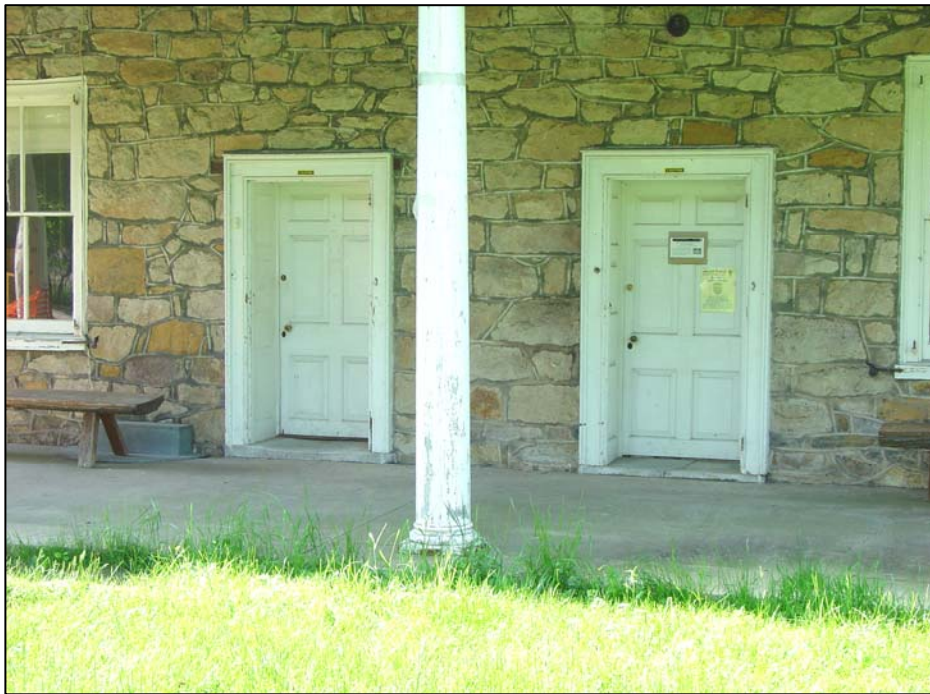
Figure 29. North elevation of the main house, showing the more elaborate raised- panel reveals of the west doorway (leading to the center hall), and the simple surround of the east doorway (leading to the original kitchen). (Photograph taken in 2004.)
