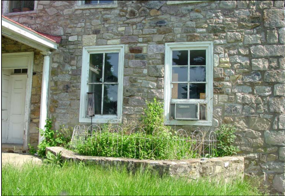
Figure 23. South elevation, east side, showing the masonry infill of the former opening for the one- story bay window, and the remaining foundation of the bay window. (Photograph taken in 2004.)
