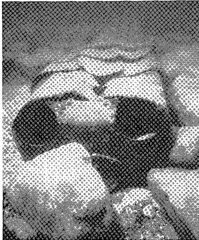
Fig. 4.30. The SUPERIOR's old-style locomotive-type boilers are built up of riveted sheets. Photo by Frederick Stonehouse.
