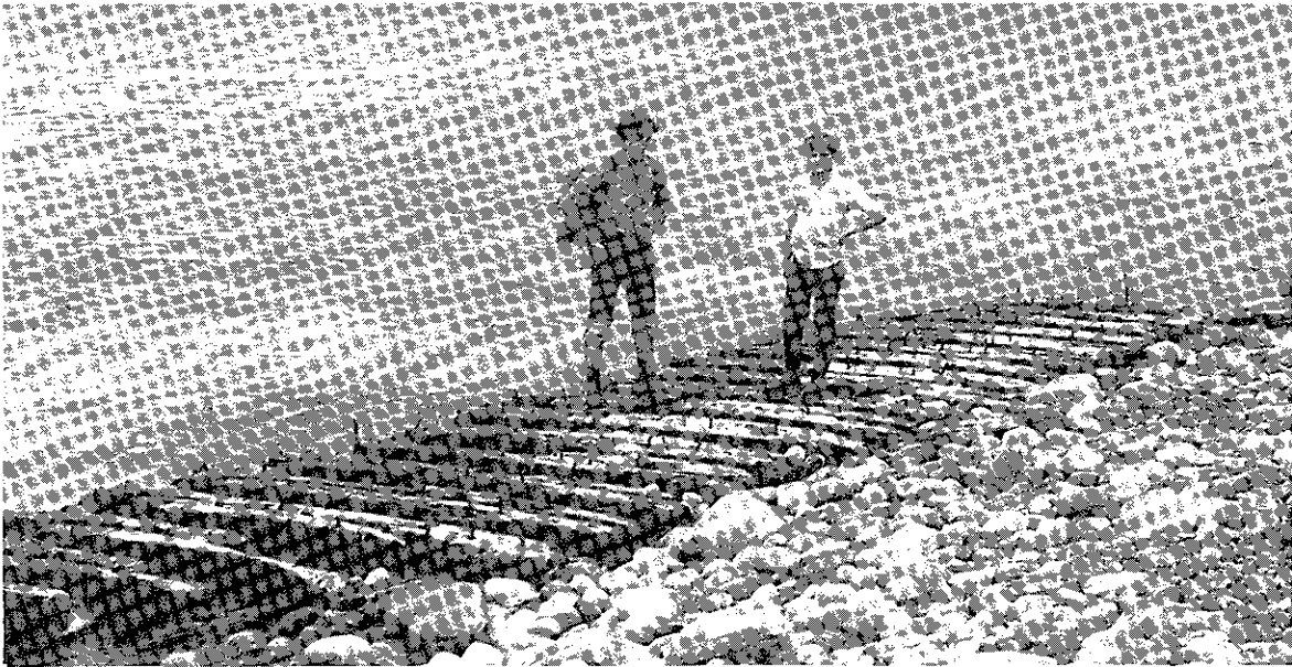
Fig. 4.43. This 1966 view shows the same section before frames were eroded by sand and gravel. Photo by Julius F. Wolff Jr.
