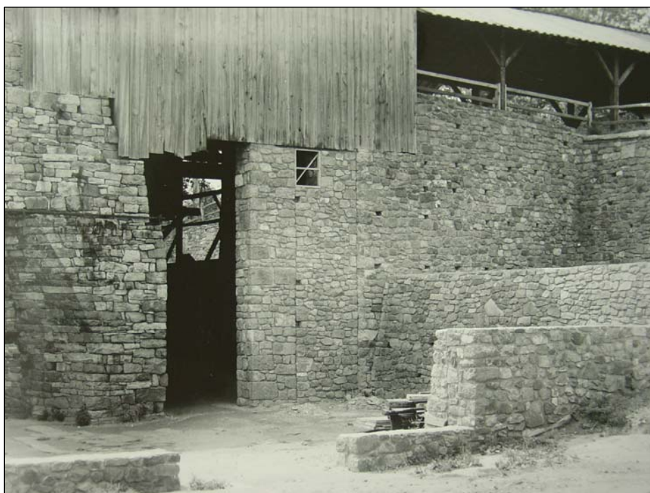
Figure 59. Partially rebuilt west wall of the cast house, north of the furnace, September 1963. The new wall is left of window below the bridge house.
