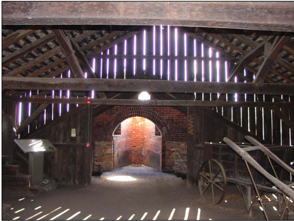
Figure 91. Interior view of the bridge house, looking south towards the tunnel-head vestibule, September 2006.
