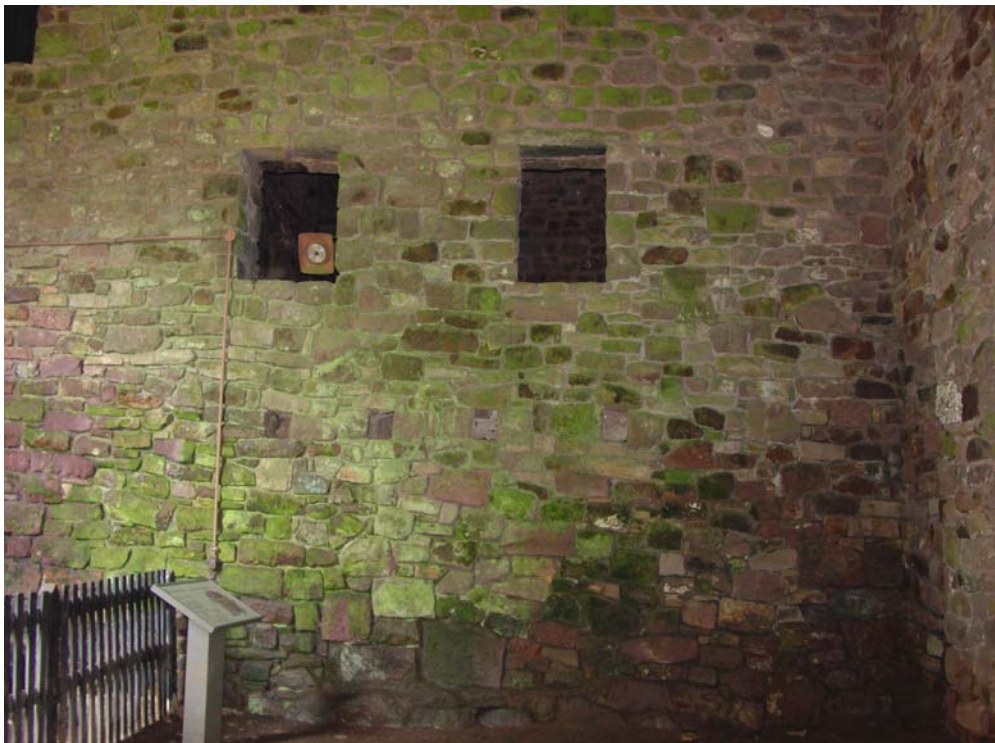
Figure 94. Reconstructed north wall ("Wall A") supporting the north end of the enclosed bridge house, July 2006.
