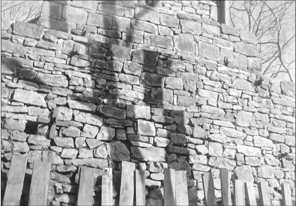
Figure 33. Detail of the west face of the furnace, showing recessed mortar joints of the completed stonework, January 6, 1939.
