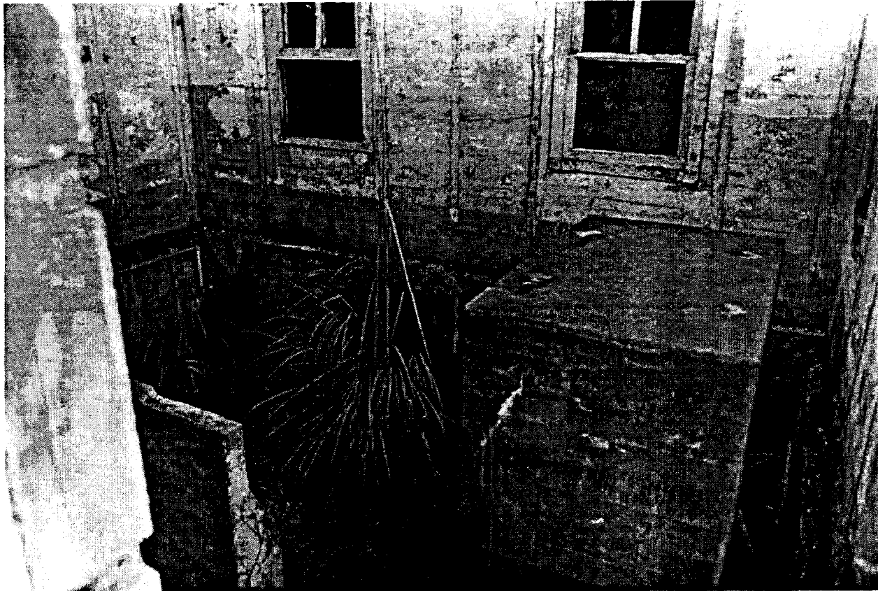
Plate 50. Absence of flooring, at the entrance to the switchboard room, mine casemate, Fort Barry.
