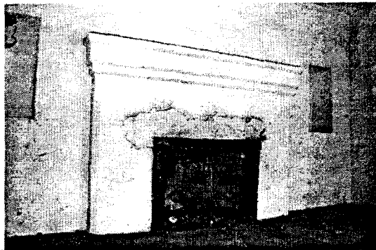
Battery Spencer. Finishwork for the fireplace in the commanding officer's room. Dependent structure.
