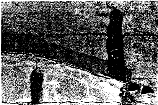
Battery Godfrey. Cold joint displaying sheet lead as waterproof layer. Stained concrete from imbedded metal elements.
