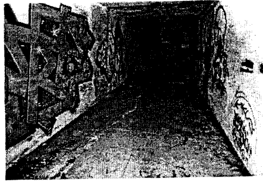
Battery Dynamite. Graffiti in cross-gallery, looking toward entry doors for emplacement one. Also showing significant floor deflection as a result of seismic action.
