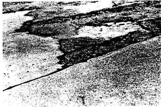
Battery Godfrey. Surface drainage system on blast apron composed of pipe, earth fill, and asphalt or oil-saturated earth.
