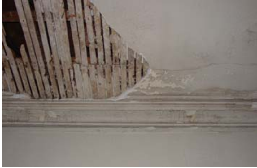
Figure 46. Officers Club, second- story center hallway (Room 201), ceiling plaster on wood lath, 2005.
