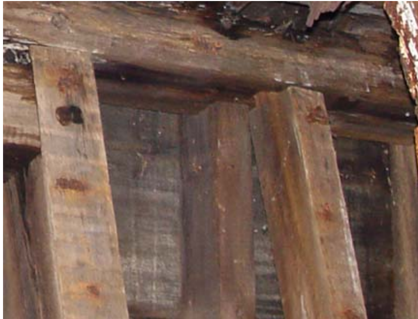
Figure 41. Officers Club, attic framing detail, showing joinery of wall stud and jack rafter into upper plate of mansard roof, 2005.
