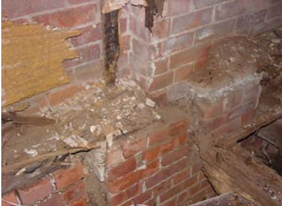
Figure 38. Officers Club, showing exterior bearing- wall construction at transition from first story to second story; also shows pockets in masonry for framing, 2005.
