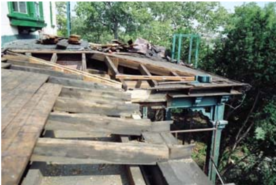
Figure 35. Officers Club, east facade, piazza roof, showing original framing with extended rafters for integral gutters.
