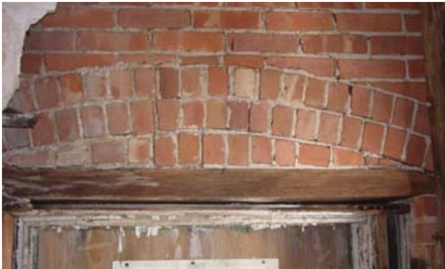
Figure 39. Officers Club, typical brick relieving arch above window opening, as seen from Ladies' Lounge (Room 103), 2005.
