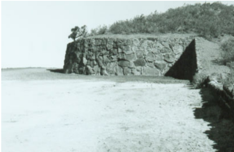
Fig. 7.20 Completed Crater Rim Retaining Wall, Circ. 1961, Photographer unknown, Completion Report, (Capulin: Capulin Volcano National Monument Administrative Records, Completion Reports), File D2621.
