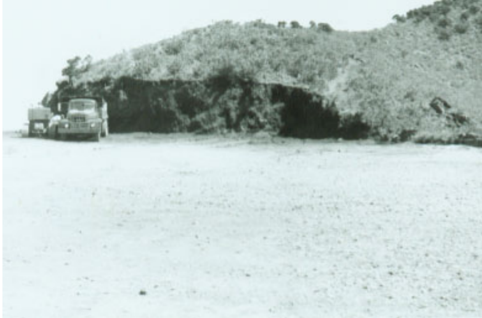
Fig. 7.19 Crater Rim Excavation for Retaining Wall, Circ. 1961, Photographer unknown, Completion Report, (Capulin: Capulin Volcano National Monument Administrative Records, Completion Reports), File D2621.
