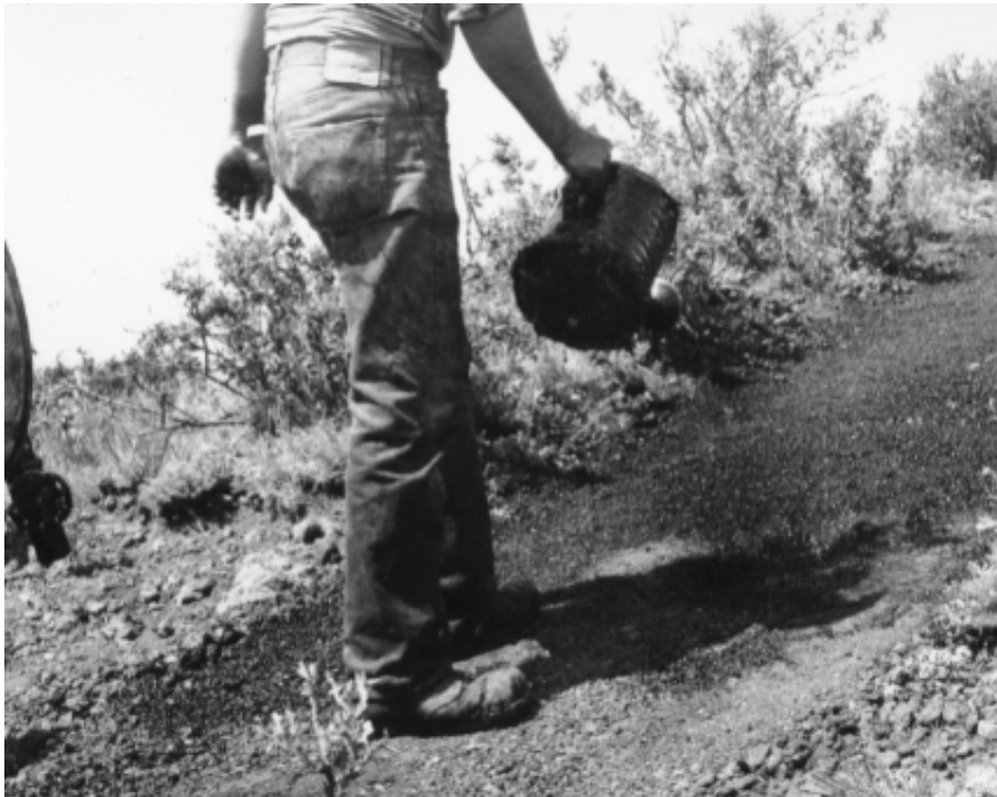
Figs. 7.26 and 7.27 Trail Reconstruction and Resurfacing, Circ. 1962, Photographer unknown, Completion Report, (Capulin: Capulin Volcano National Monument Administrative Records, Completion Reports), File D2621.
