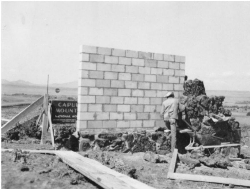
Figs. 7.36 & 7.37 New Entrance Sign Construction, Circ. 1964, Photographer unknown, Completion Report, (Capulin: Capulin Volcano National Monument Administrative Records, Completion Reports), File D2621.
