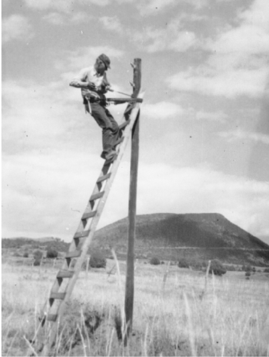
Fig. 7.31 Putting up Poles and Stringing Wire, Circ. 1963, Photographer unknown, Completion Report, (Capulin: Capulin Volcano National Monument Administrative Records, Completion Reports), File D2621.
