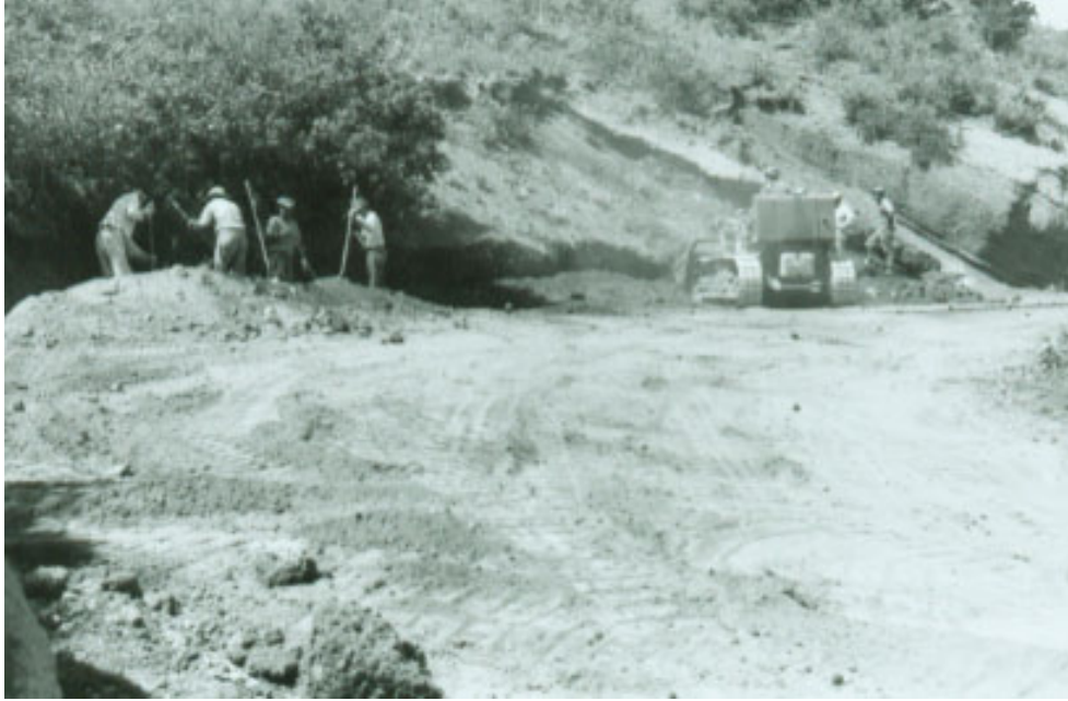
Fig. 7.21 Excavation for Additional Crater Road Retaining Wall, Circ. 1961, Photographer unknown, Completion Report, (Capulin: Capulin Volcano National Monument Administrative Records, Completion Reports), File D2621.
