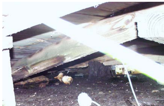
Figure 25 View of collapsing floor under Room 104. (NPS-SERO-CR, 2002)
