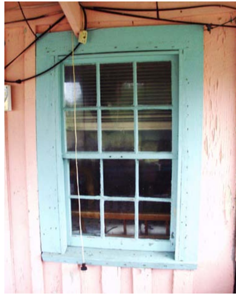
Figure 29 View of window W-2 on southeast (front) side of house, with exterior siding and trim typical of the original building. (NPS-SERO-CR, 2002)
