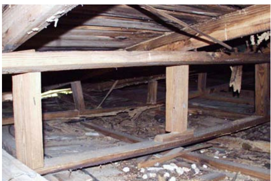
Figure 28 View of heavily-damaged roof and ceiling structure over Room 104. (NPS-SERO-CR, 2002)
