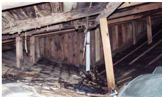
Figure 26 View of junction of roofs of two original structures; note severe termite damage in rafters and decking at left. (NPS-SERO-CR, 2002)
