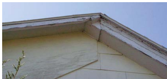
Figure 25 View of typical boxed cornice at right and modern alteration to front shed of roof at left. (NPS-SERO-CR, 2003)
