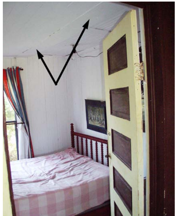
Figure 32 View east in Room 102, with arrows indicating line of wall that was relocated to create this room. (NPS-SERO-CR, 2003)
