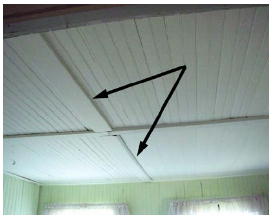
Figure 30 View of ceiling in Room 101, with arrows indicating location of wall that originally divided the space. (NPS-SERO-CR, 2003)
