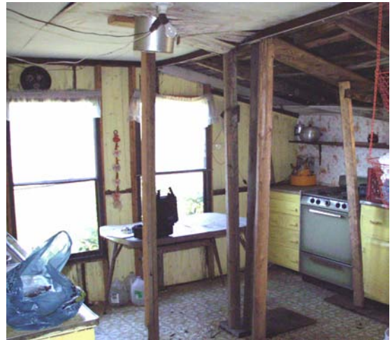
Figure 35 View west in Room 103, showing deteriorated shed-roofed addition that was combined with this room after World War II. (NPS-SERO-CR, 2003)
